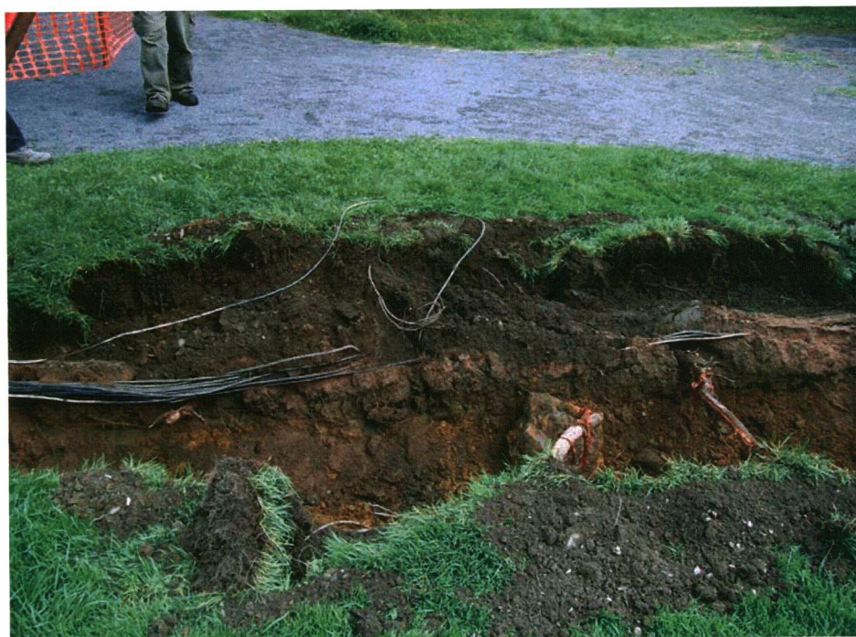
Plate 2: East wall profile of catch basin trench showing the previously-excavated electrical trench.
