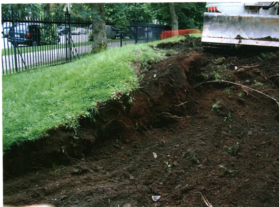
Plate 1: Excavation of artificial berm to west of park entrance on Spring Garden Road, looking southwest.
