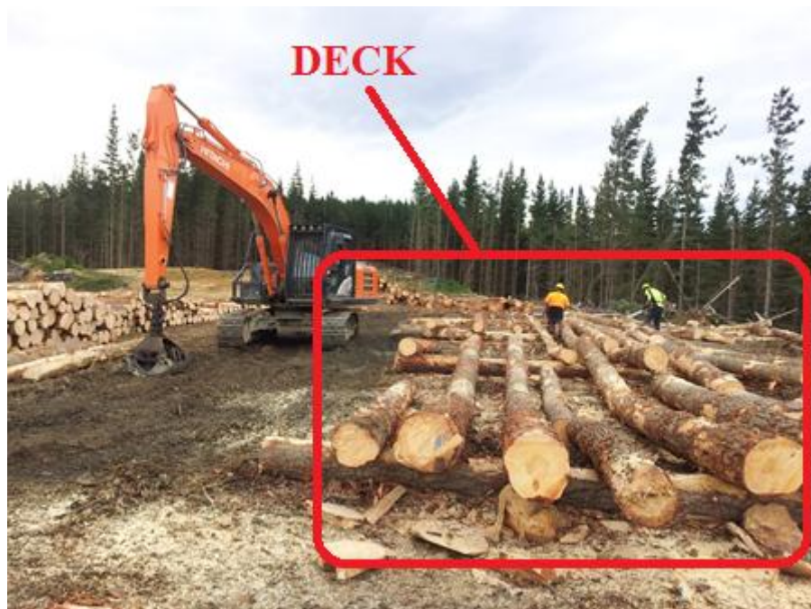
Figure 2 - Example of the processing area of a landing known as a ‘Deck’.
