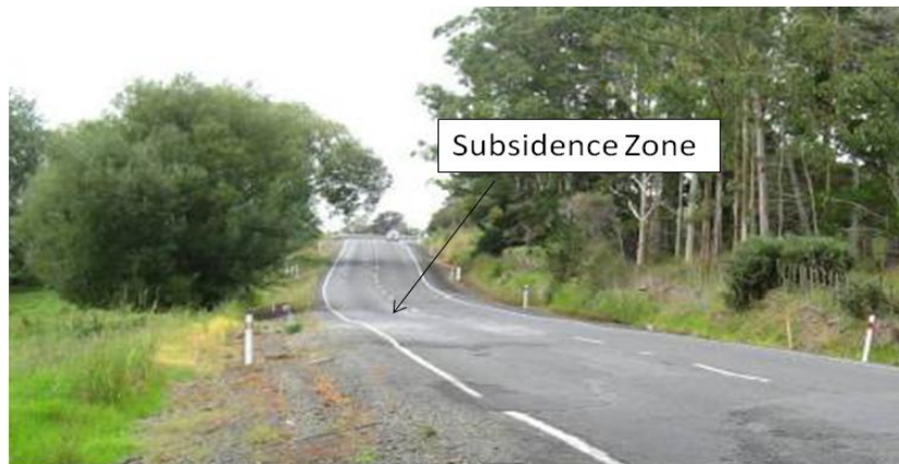
Figure 6-3: Deformation in road carriageway and subsidence of embankment (O'Sullivan, 2009).
