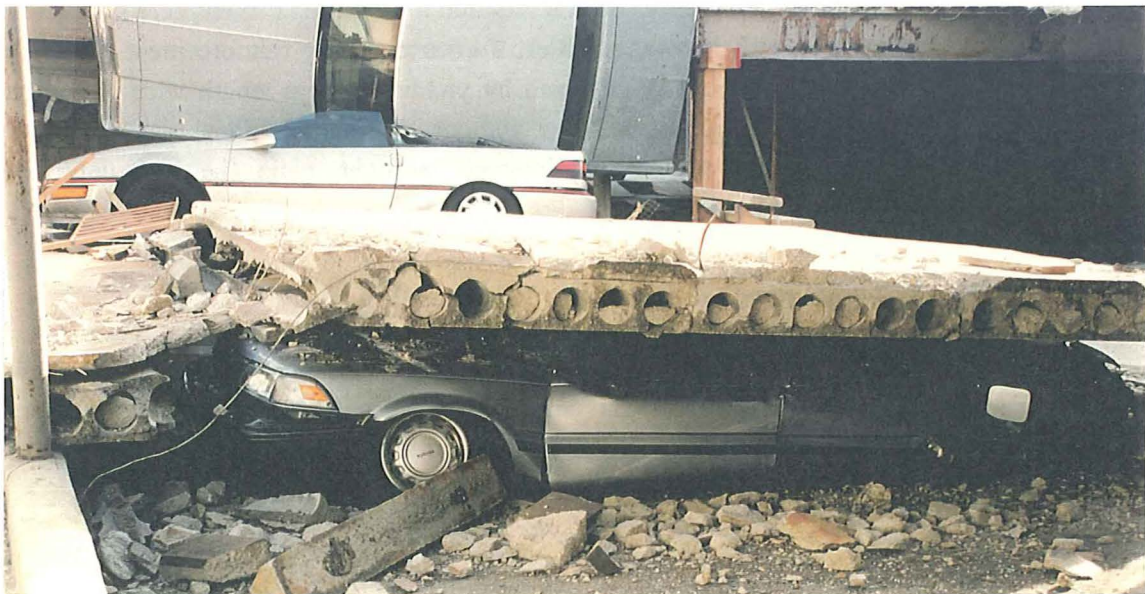
Fig 1.64 Failure of a single storey car park floor at Northridge
