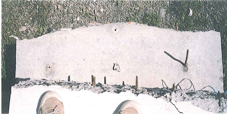
Fig. 3.27 End view of hollow core unit, showing inclined planes of fracture caused by combined shear and tension at the support
