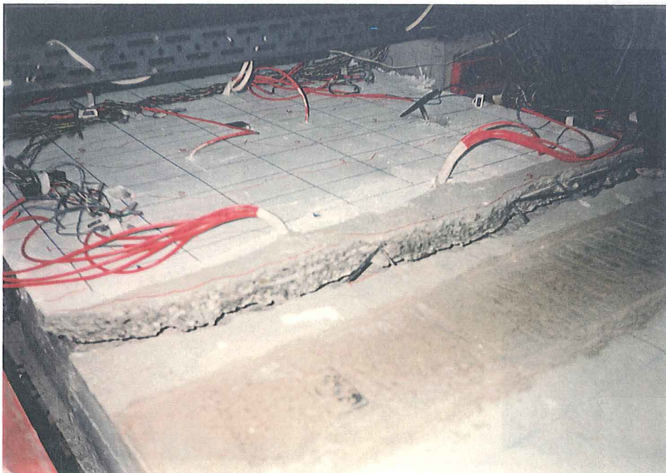
Fig. 3.23 Separation of the principal topping crack immediately prior to collapse
