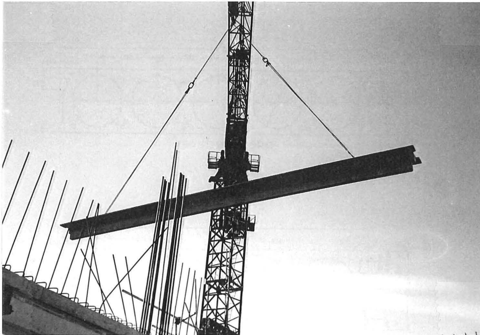
Fig. 1.8 Single tees used in the construction of the new Civil and Mechanical Engineering buildings at the University of Canterbury School of Engineering (1996).
