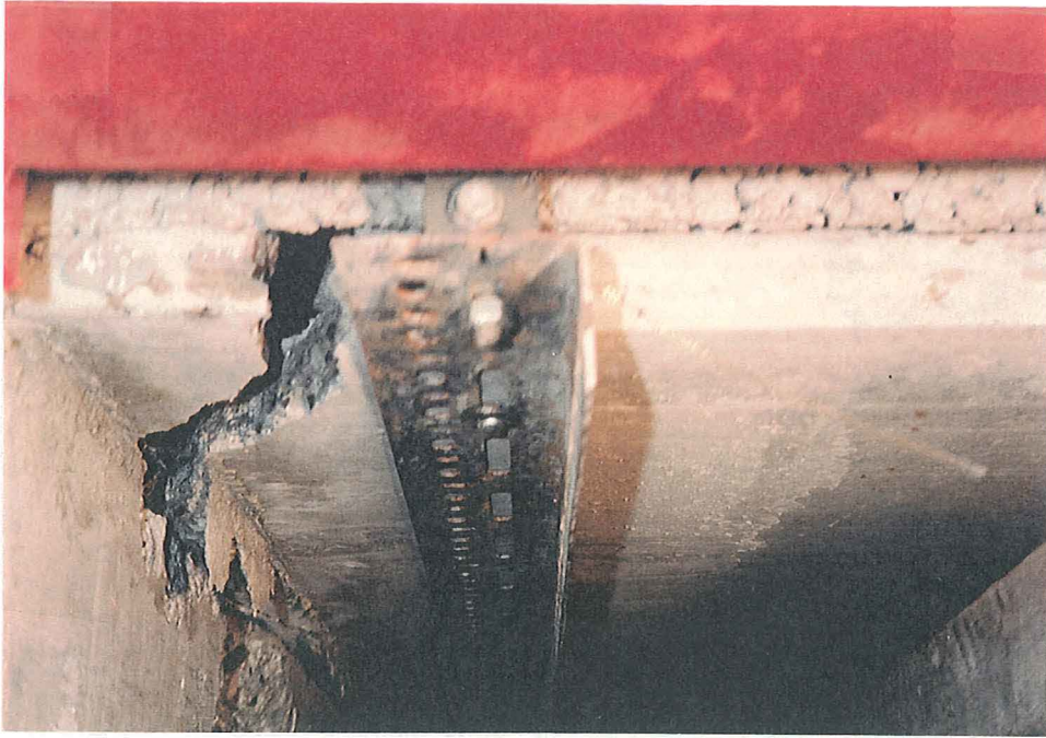
Fig. 3.22 Soffit of hollow core unit showing fracture at the support
