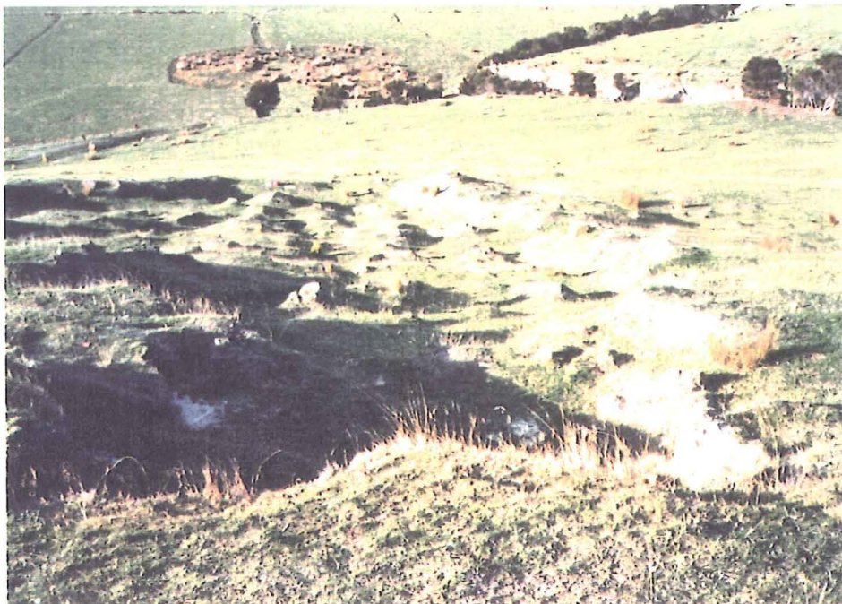
Figure 3.12 Drainage Channels in Investigated Failed Ground Complex. Note smoothing of slope features, resulting from the erosional action of surface runoff water.
