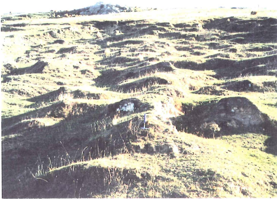
Figure 3.9 Terracette like Slump Features within Investigated Failed Ground- looking upslope.
