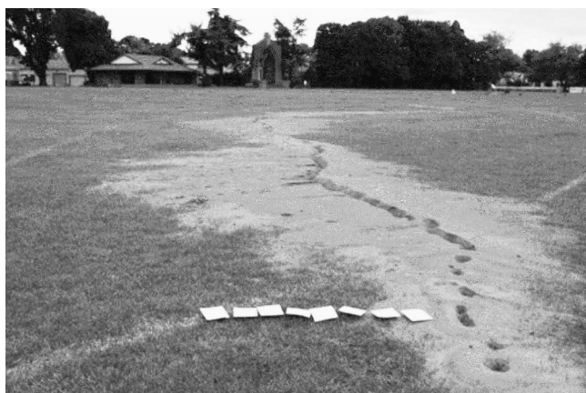
Figure 2. Photograph of one of the “silt volcanoes” caused by liquefaction at the CBHS site before removal of the ejected silt. Note that the mound is elongate in the WNW-ESE direction, in this case, and has a narrow vent. (Photograph courtesy of S. Dods of CBHS). No photo of the piston failure before remediation is available.
