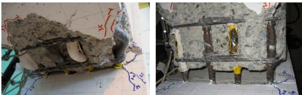
(a) Buckling at -3.5 % drift
