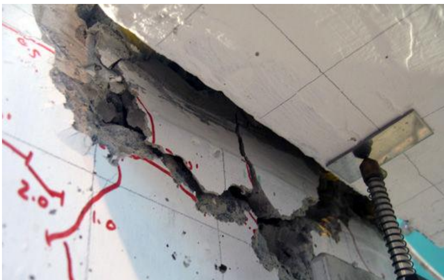
Figure 2-16: Concrete cone pullout on face of beam-column joint specimen SB2 (Au, 2010)
