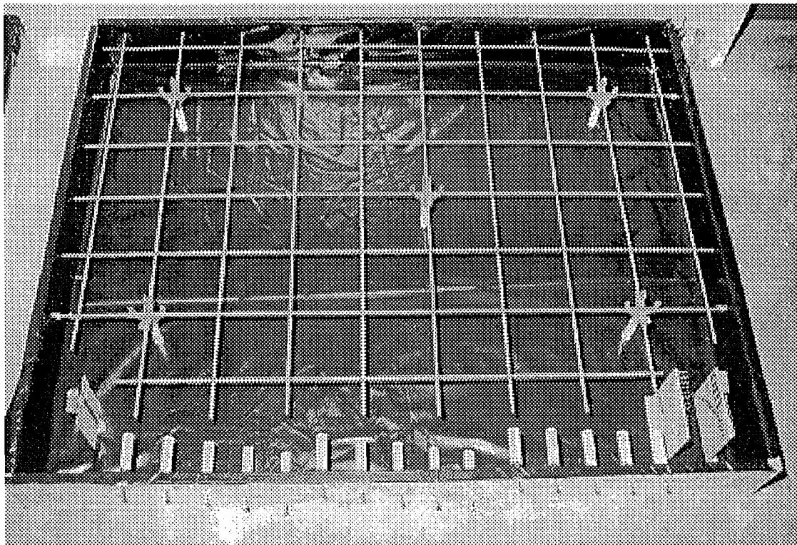
Figure 4.3-3: Slab #5 before pouring, showing the reinforcing mesh and the positions of the horizontal electrode systems (from left to right, HES#1, HES#3 and HES#2).
