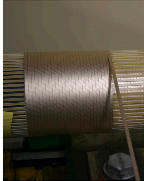
(b) The second layer being wound, showing the inter-layer insulation.
