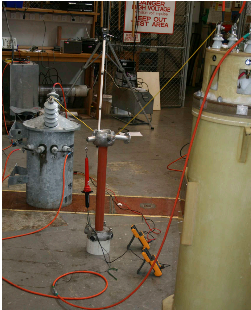
Figure 6.11 Photograph of the test setup for the separate source ac withstand voltage test.
