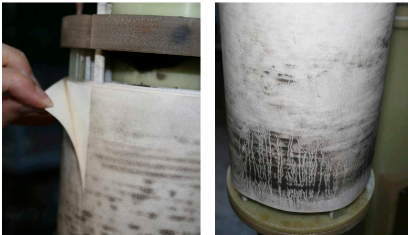
(a) The contaminants appear only on the outside of the insulation. (b) The contaminants found on the lower portion of the windings.
