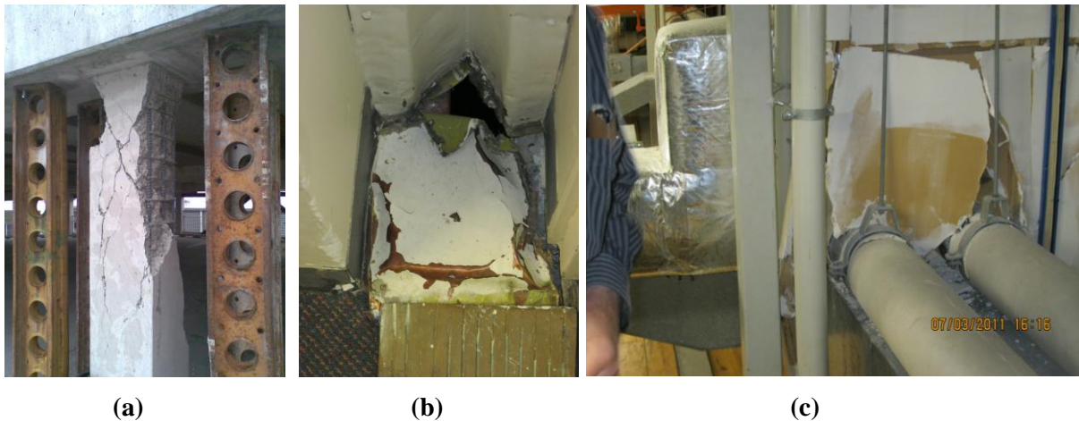
Figure 2. Observed structural damage in non-clinical and clinical buildings: a) spalled concrete in ground-floor column of a parking structure, b) separation joint damage in Riverside Building, and c) damage to firewalls in the CWH (photo credit, Alan Bavis).
