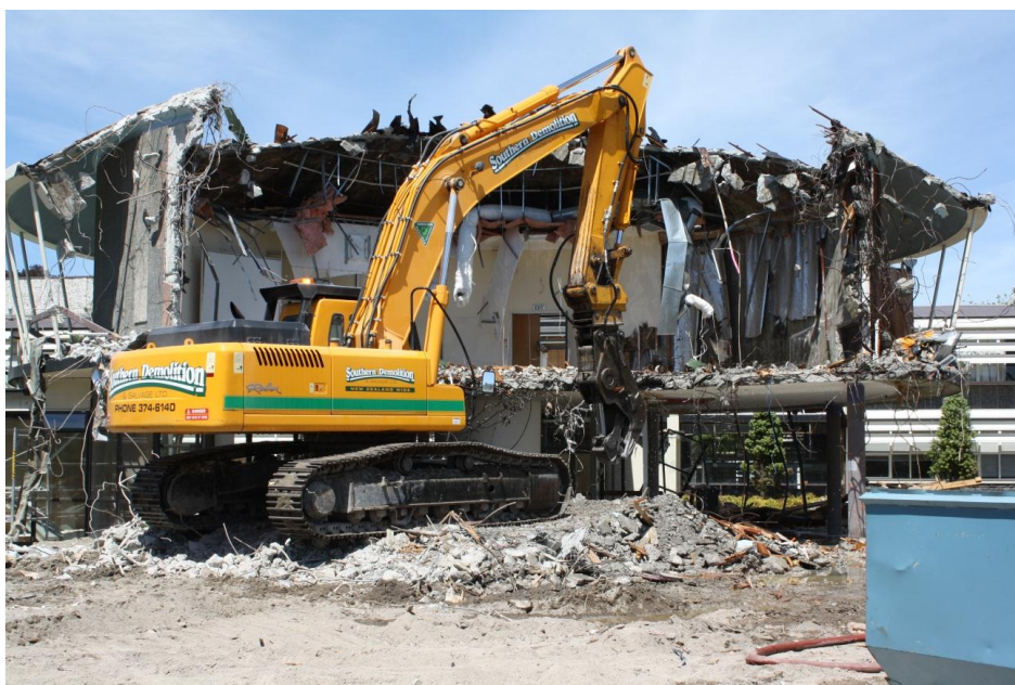
Figure 3-9 Demolition of the University of Canterbury, Engineering School “Mushroom”. (Photo date: December 2011.)
