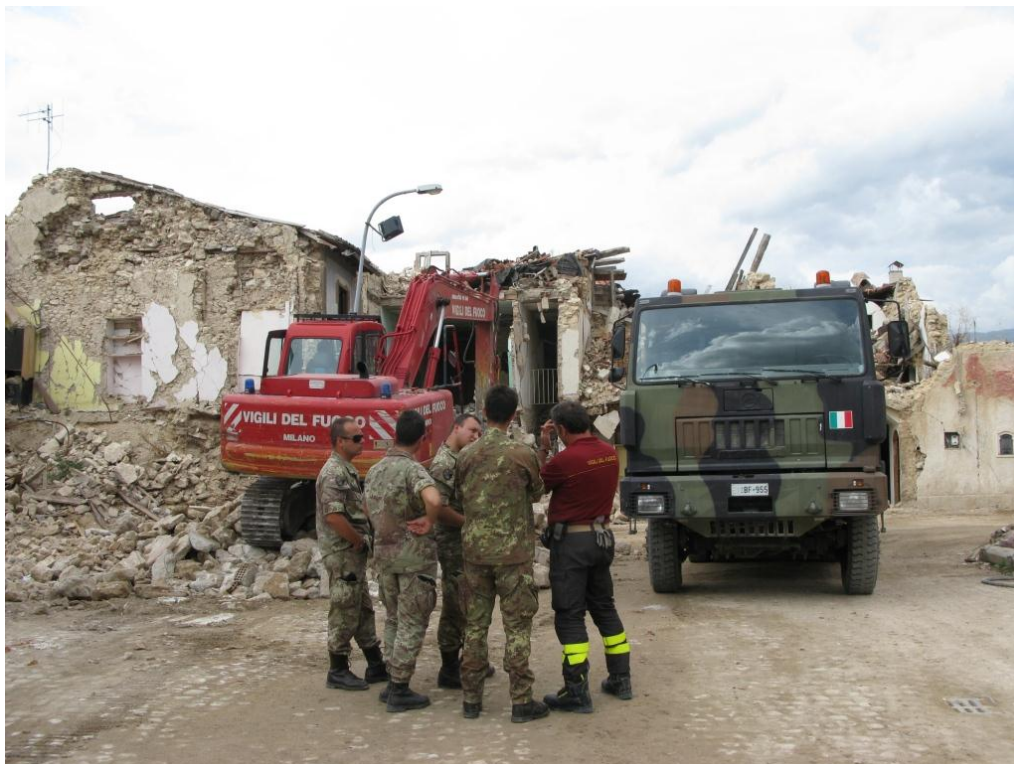
Figure 3-4 Fire Service and Army personnel carry out demolition of houses in Onna, one of the towns most affected by the 2009 L'Aquila earthquake; September 2010.
