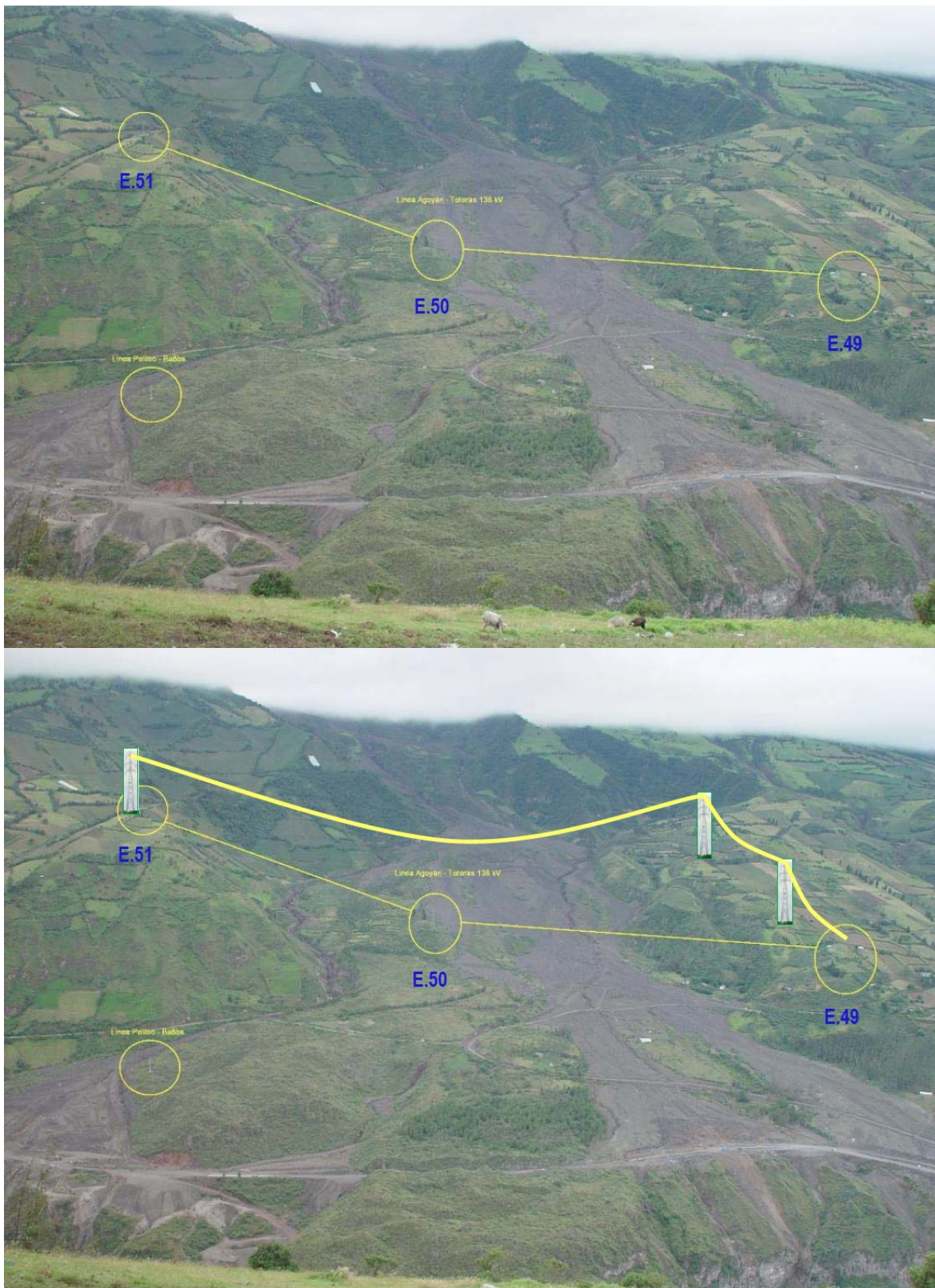
Figure 14 Above: 138 kV transmission tower (E50) situated in a 2006 lahar path. Below: Proposed re-design of the 138 kV transmission circuit showing relocation of towers and conductors (lines) to avoid lahars (Photo's courtesy of Transelectric, Ecuador).
