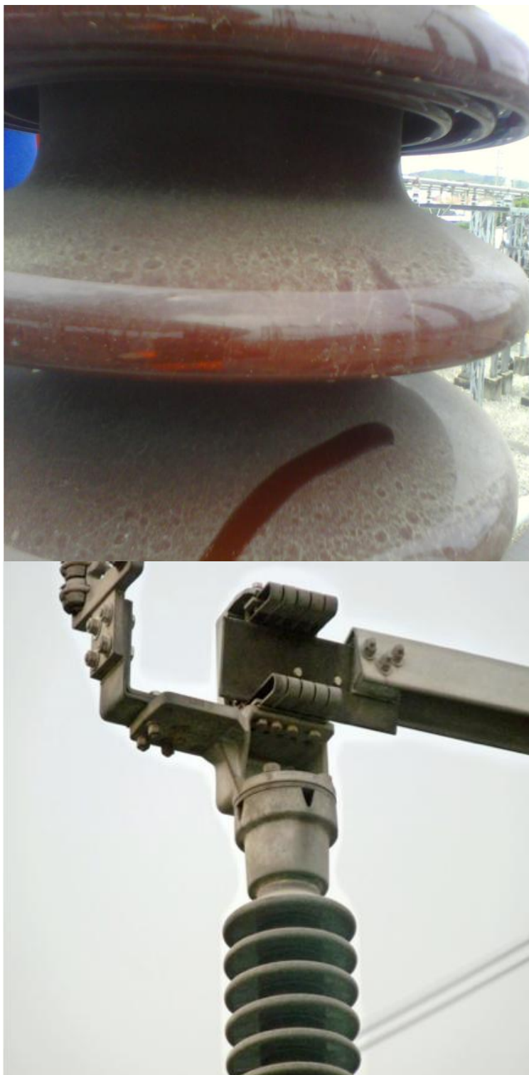
Figure 13 Above: 138 kV transformer bushing coated in 1-2 mm of fine-grained ash at a Guayaquil substation. Below: a contaminated disconnect switch. (Photos Courtesy of Transelectric, Ecuador).
