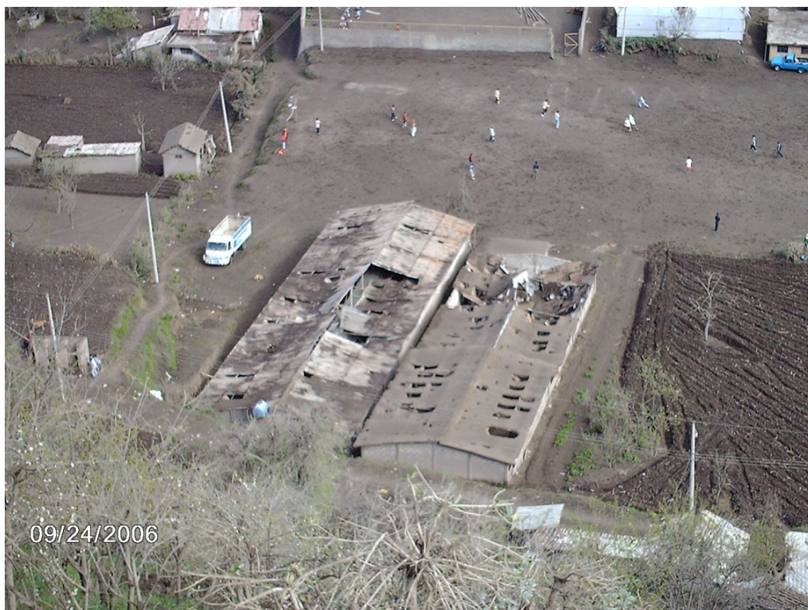
Figure 19 Ballistic block damage to shed roof, Cotaló, 2006 (photo courtesy of Carlos Fernando Perez).
