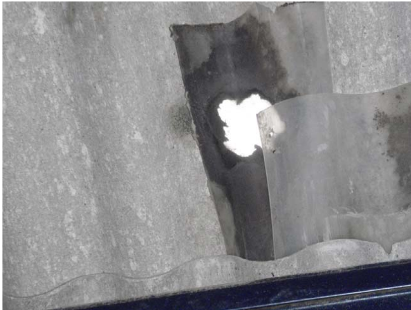
Figure 22 Ballistic damage to the roof of a chicken shed.
