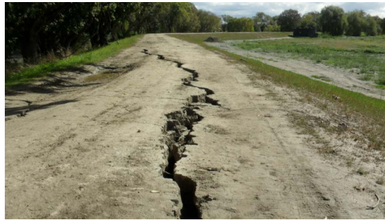
Figure 5. Example of longitudinal cracks running along the crest of the levee.
