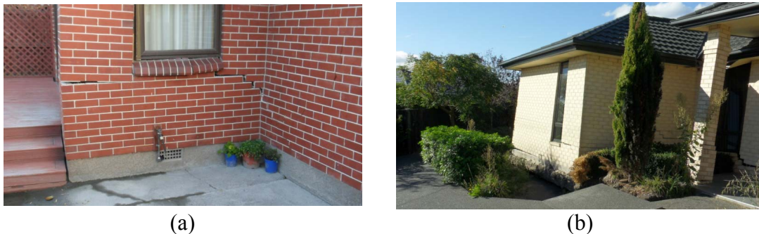
Figure 2. Examples of liquefaction damage to houses in: (a) Hoon Hay with differential settlement, and (b) south Kaiapoi with lateral spreading.
