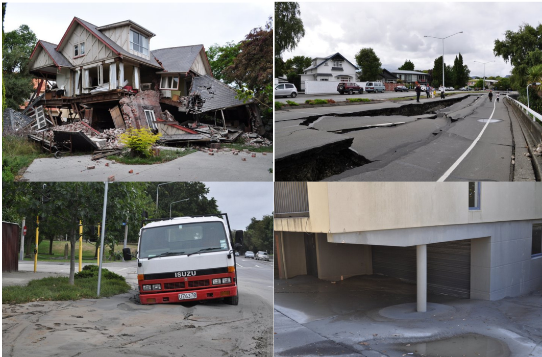
Figure 1.1: Severe damage to Christchurch CBD from the February 2011 earthquake of magnitude 6.3 ML: top-left) collapse of residential buildings, top-right) extensive damage to roads, bottom-left & -right) widespread liquefaction around the city (Photos courtesy of Mohammad S. Ashtiani)
