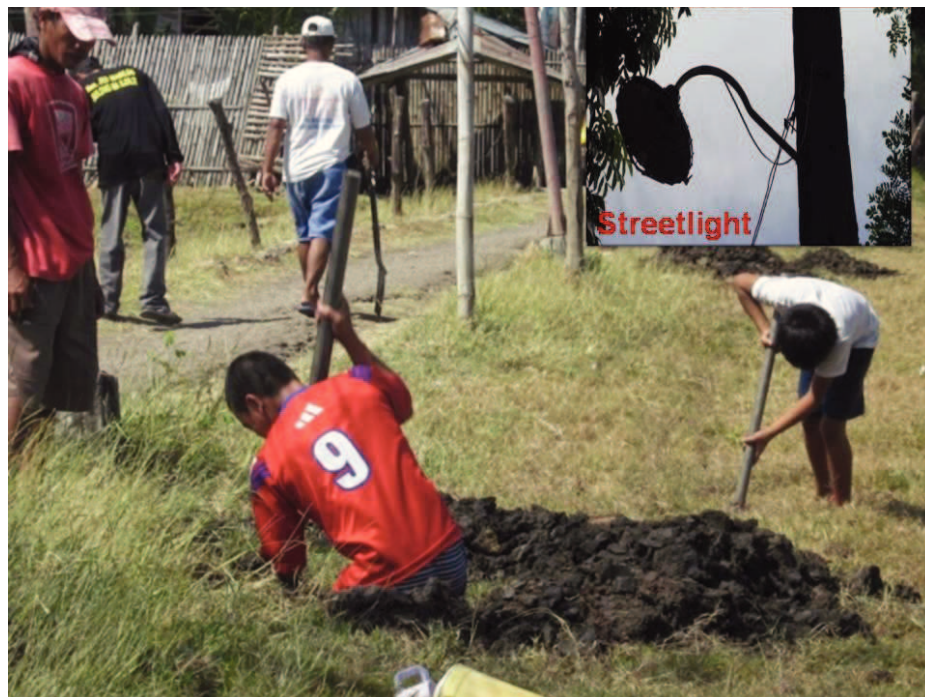
Figure 5.5 Streetlight project during construction. Inset photo shows one of the streetlights (Photo: HPFP, 2008; Text: Author).
