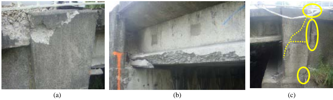
Figure 13: Fitzgerald Avenue Bridge. Pounding damage (a) at the abutment, (b) to the immediate adjacent girder and (c) to the other abutment.
