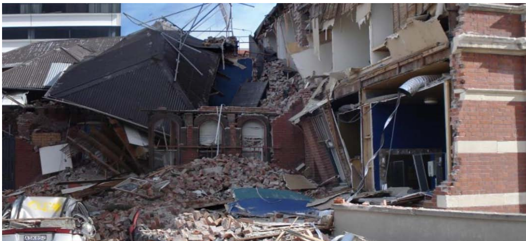
Figure 8: Two storey building collapse involving pounding. Primary cause of collapse is attributed to URM construction
