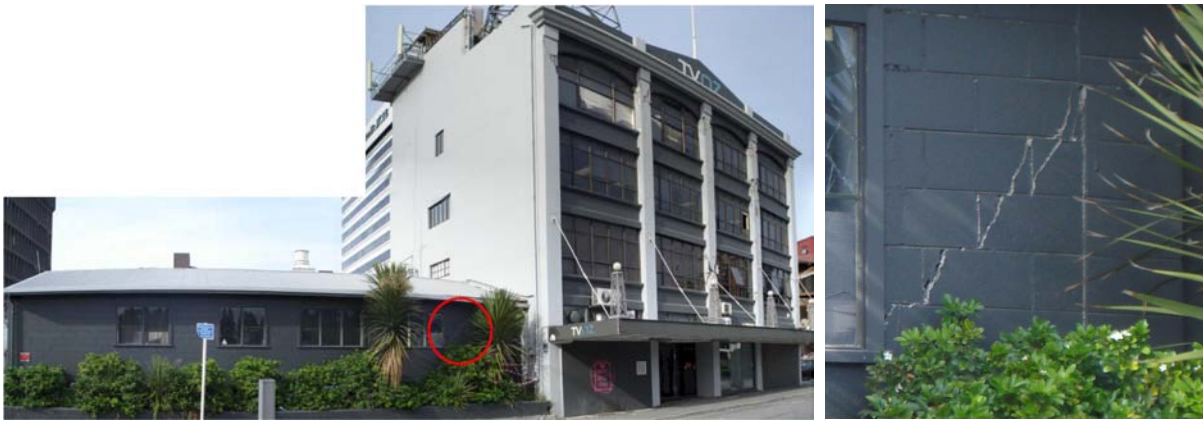
Figure 7: Pounding between 1 storey and 4 storey buildings. Damage to four storey building not attributed to pounding
