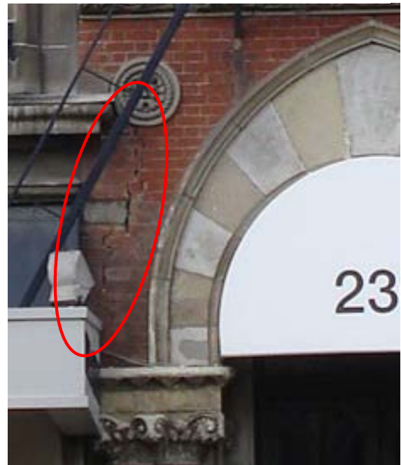
Figure 9: Masonry damage after the Darfield earthquake
