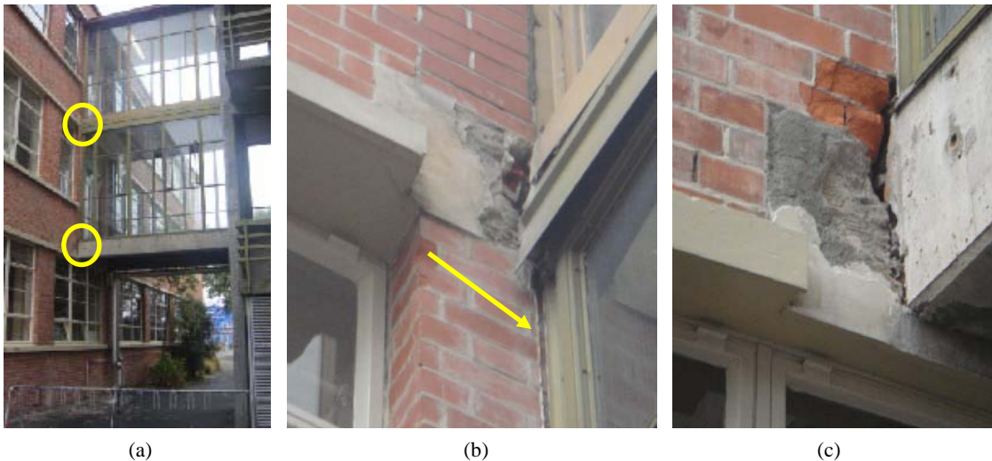
Figure 11: Pounding damage to buildings at the Christchurch Polytechnic Institute of Technology. (a) Adjacent buildings with pedestrian bridges, (b) upper and (c) lower pounding locations.
