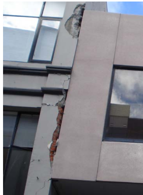
Figure 6: Damage between central and rightmost building
