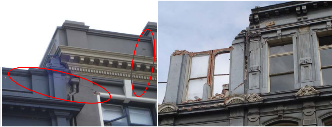
Figure 1: Examples of URM pounding damage. Left: minor damage. Right: major damage partially caused by pounding
