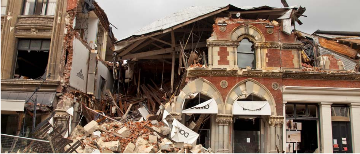
Figure 10: Building collapse involving building pounding. Primary cause of collapse is attributed to URM construction. Photo courtesy of Colin Monteath, Hedgehog House.
