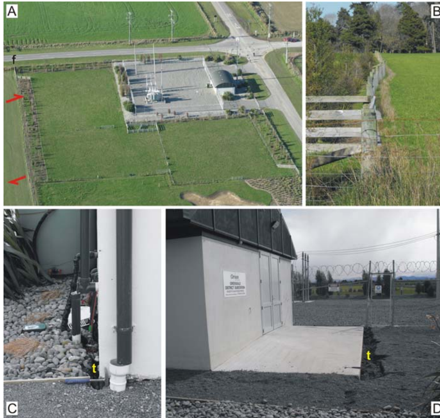
Figure 6. A) Light-industrial building with a reportedly well-reinforced concrete slab foundation is tilted and rotated, but relatively undamaged, by \sim 1.7 m dextral and < 1 m vertical (south side up) displacement distributed across a \sim 100 m wide deformation zone. Red arrows denote location, strike and sense of lateral displacement of the surface rupture deformation zone. Photo by Richard Jongens looking NE. B) Fence line adjacent to site crosses the surface rupture deformation zone and records the amount, width, and distributed style of fault displacement here (camera location for B is shown by black “f” in A). Photo by Russ Van Dissen looking SW. C & D) Long axis of building is oriented \sim 55^\circ counter-clockwise to the general strike of the fault rupture. Distributed displacement imposed tensile ground strains across the site with an orientation roughly sub-parallel to the building’s long axis. The foundation of the building was robust enough to resist these strains (i.e. no cracking of the foundation was evident) and, instead, the soil pulled away from either end of the building’s foundation (yellow “t” in C & D). Photos C & D by Russ Van Dissen looking NW.
