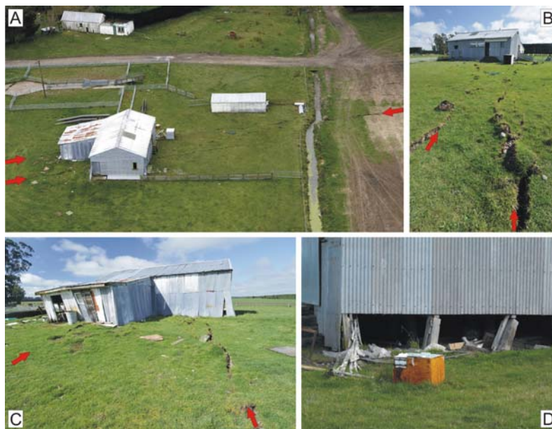
Figure 5. Timber-framed farm shed that is located within a 25 to 50 m wide deformation zone comprising both discrete shears (red arrows) and distributed deformation, and accommodating ~2.7 m of net slip (predominantly strike-slip - note dextral offset of irrigation channel in right-hand side of A). The farm shed is made up of two parts, a larger metal-clad structure with a timber floor that is founded on shallow seated ~700 mm high concrete piles (D), and a smaller lean-to structure attached to the side (A & C). The lean-to is a pole building (part metal-clad and part wood-clad) with an unreinforced concrete floor. The response of the two different construction styles to surface fault rupture was noticeably different. The support poles of the lean-to are set into the ground. Dextral fault rupture under the lean-to led to lateral displacement of the support poles on either side of the rupture, and significant distortion of the walls and roof (C). In contrast, surface rupture deformation under the larger piled structure was, in large measure, isolated from the superstructure by rotation of the shallow seated piles. The timber flooring and framing, and metal cladding proved a resilient structural system that limited internal distortion. It would be a relatively straightforward process to re-level and reinstate this portion of the building. Photos: A by Richard Cosgrove looking NE; B by Dougal Townsend looking W; C by Dougal Townsend looking E; D by Russ Van Dissen looking SW.
