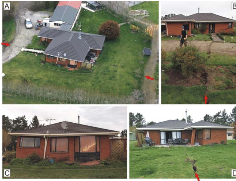
Figure 4. Timber-framed, brick-clad house with concrete slab foundation (at most only lightly-reinforced) and light-weight roof that is located within a ~150 m wide deformation zone accommodating 4 to 5 m of dextral displacement. The house is badly damaged by distributed deformation, and ~0.5 m of discrete strike-slip rupture (red arrows) that enters the house through the front door (B), passes through the house's foundation (including living room), and exits through the back door (D). Photos: A by Richard Cosgrove looking S; B by Hayden Mackenzie looking WNW; C by Hayden Mackenzie looking SSW; D by Dougal Townsend looking ESE.
