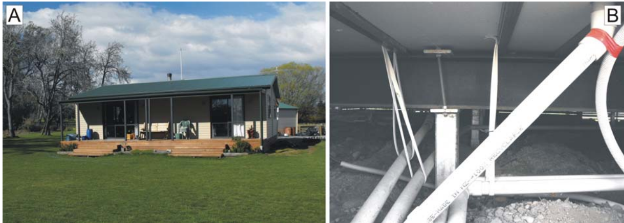
Figure 7. A) Light-gauge steel-framed, plywood- and weatherboard-clad house with steel pile foundation, steel I-beam bearers, steel joists and plywood flooring that is tilted, and rotated, but only slightly damaged by ~1 m of distributed vertical and dextral fault rupture spread over several tens of metres width. Photo by Russ Van Dissen looking E. B) Close-up of pile, bearer and deformed bolted connection. Photo by Russ Van Dissen looking WNW. Despite this house being essentially “locked” into the ground (piles are concreted to ~1 m depth into the ground), it suffered only slight damage because surface rupture deformation was distributed and relatively evenly spread across the site, and because the structural system was strong and stiff enough to tilt and rotate as a rigid body. Given this structure’s resilient, and somewhat uncommon, construction style, it should be a relatively straightforward process to re-level and reinstate the house. This building was subjected to both surface fault rupture and epicentral-strength strong ground shaking, and performed in a fashion that not only greatly exceeded life-safety objectives, but will also greatly facilitate post-event reinstatement. However, if the building had been subjected to greater amounts of deformation, especially discrete displacement, the pile foundation may have been able to transfer enough deformation into the superstructure to damage it. Design modifications to potentially mitigate this, yet still retain the building’s noteworthy resilience, could be to: i) use piles specifically designed to yield during surface fault rupture, and/or ii) use two sets of bearers with one set attached to the piles and oriented parallel to the strike of the fault, and another orthogonal set on top, onto which the floor joists are attached. With due geological and engineering consideration both these options could conceivably be employed to successfully isolate ground rupture from the superstructure and still retain the advantageous ease of re-leveling qualities of this type of construction.
