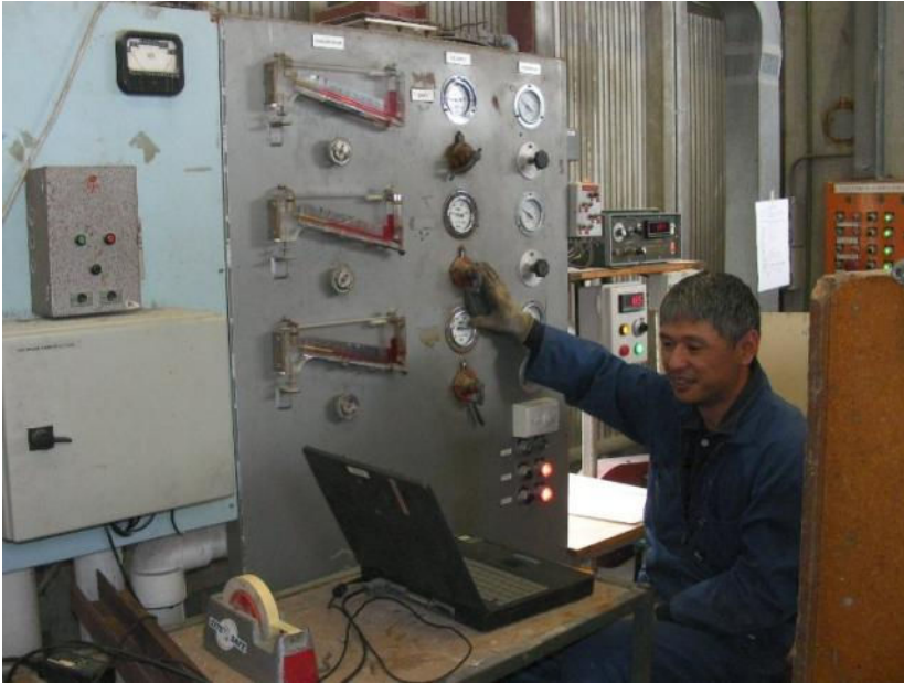
Figure 5-2: Pilot furnace control panel
