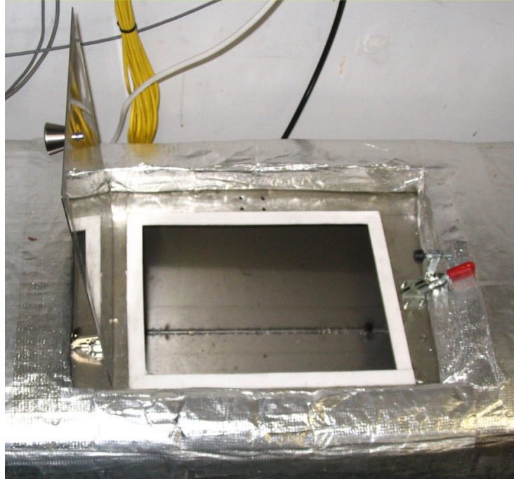
Figure 9: Hatch to admit inlet air
