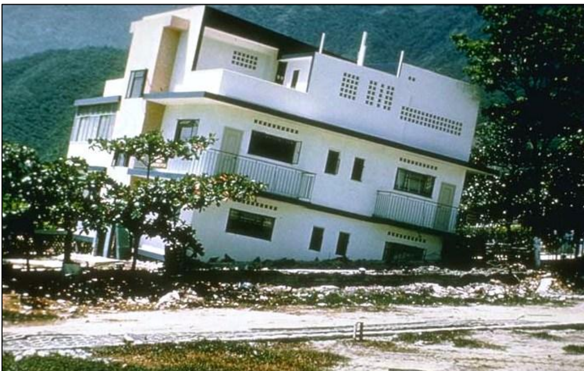
Figure 3.2: Tipped residence due to differential settling, Caracas, Venezuela (US National Geophysical Data Center (NGDC) 1967).
