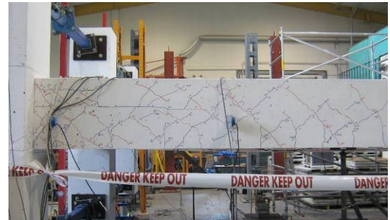
(h) Torsional cracks in the transverse beam
