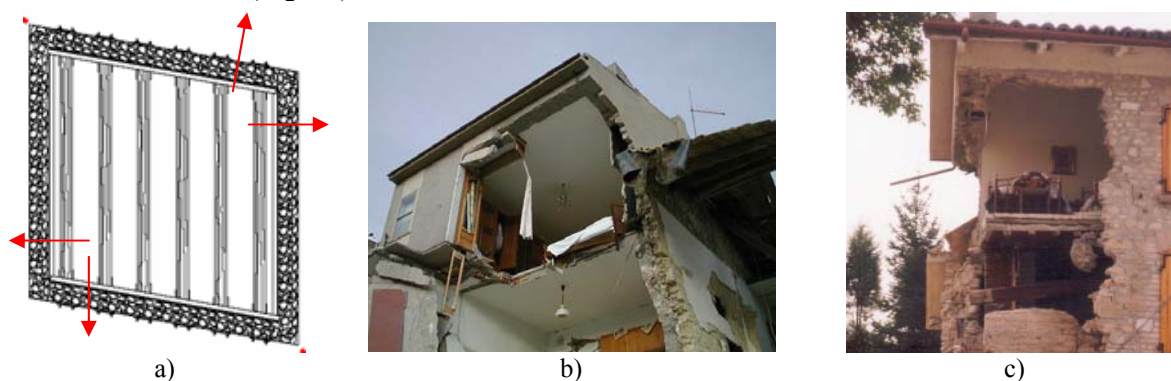
Figure 6. Angular deformation of the masonry unit and expulsion of the building corners.
