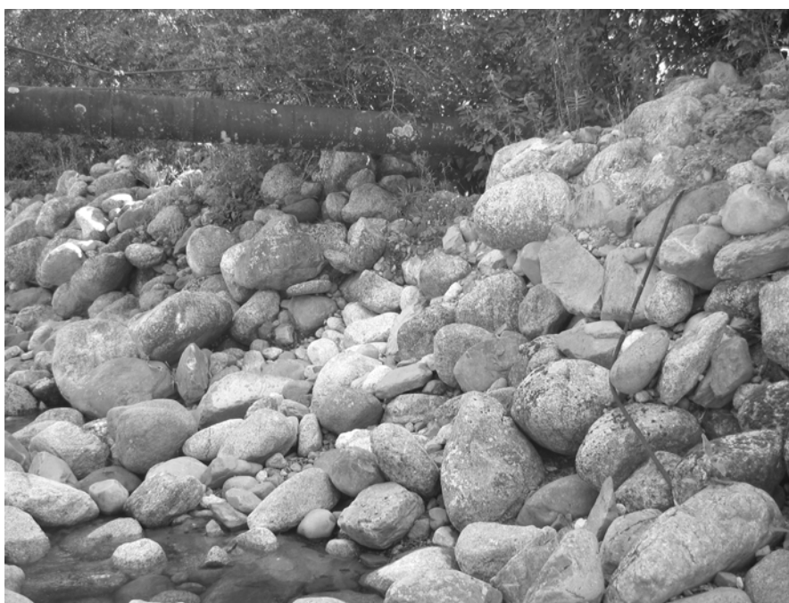
Figure 3: Debris flow levee with partially buried cable (RHS) & original pipe
