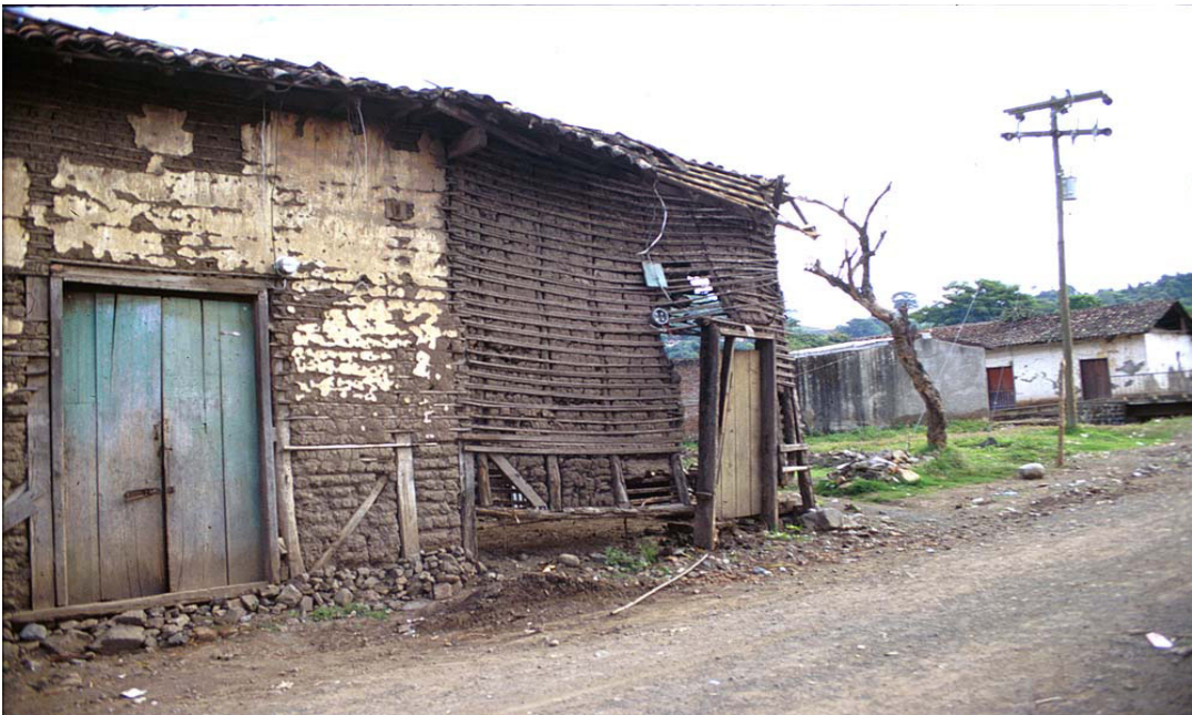
Figure 7.11 A house destroyed by the 1999 rains Source: Julie Cupples
