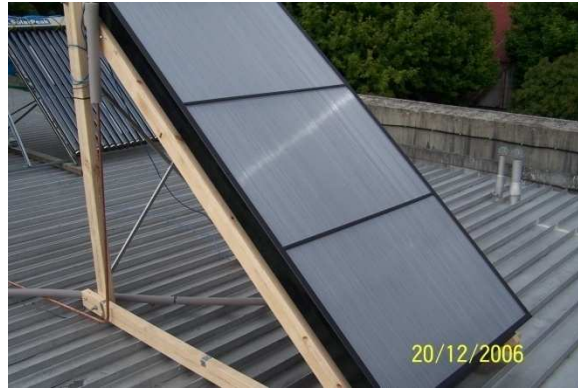
Figure 10.18. Cheap pressed steel & welded frost proof polycarbonate covered panel, December 2006.
