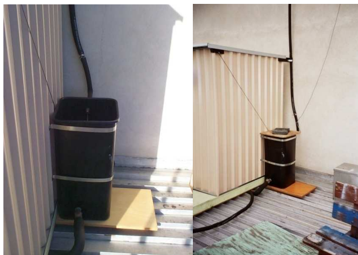
Figure 5.10 a & b. The low pressure holding tank.
