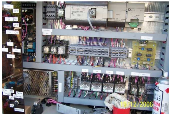
Figure 7.3. The control panel complete and in operation December 2006.
