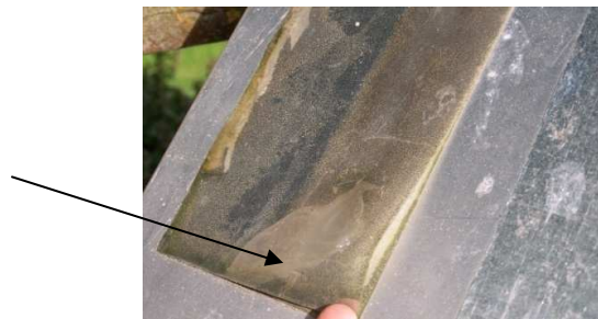
Figure 8.20 a. Delamination and lifting of 3M substrate right front edge.
