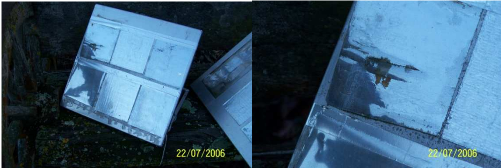
Figure 8.54 a & b. AP#2 taken 22 nd July 2006, the continuing failure of 3M substrate.
