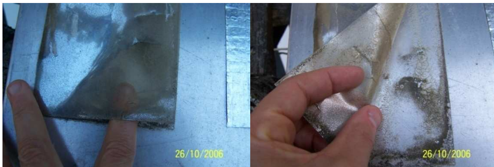
Figures 8.27 c & d. TP#2 enlarged showing top Mylar layer separation from the silver and backing material.
