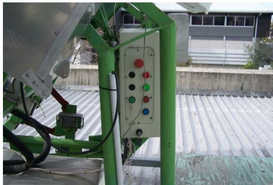
Figure 5.25. Control panel with pushbuttons and status indicators on the left-hand side of the revised control cabinet.
