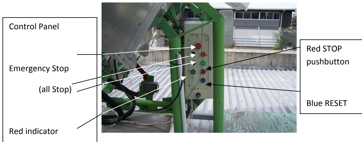
SET Control Panel
