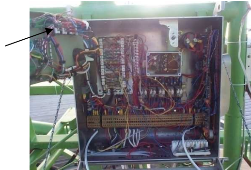
Figure 5.2. The original SET control panel with the front gear plate removed.
