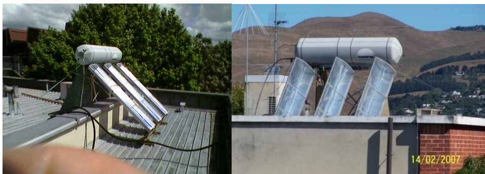
Figure 11.1 a & b. Solar trough in operation Dec 2006 (midday) and Feb 2007 (1500 hrs).
