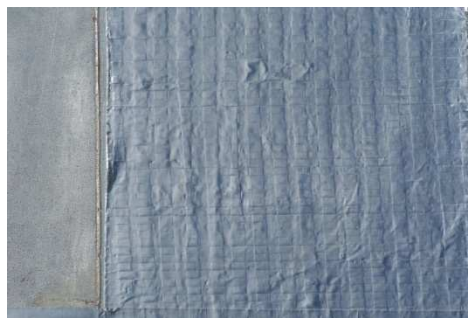
Figure 8.51 c. AP#1 taken 25 th January 2006 showing substrate failure 3M substrate.
