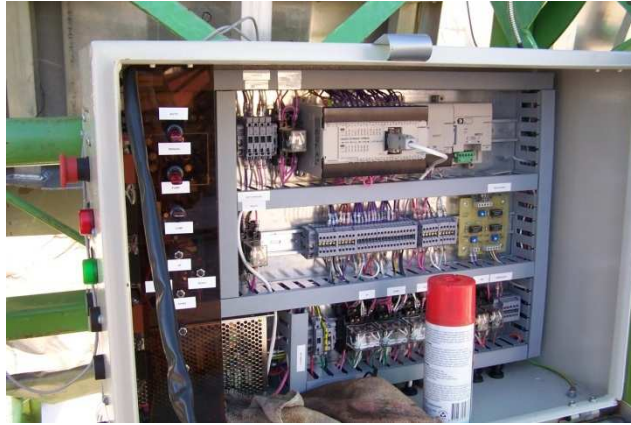
Figure 5.28. The control cabinet July 2005.
