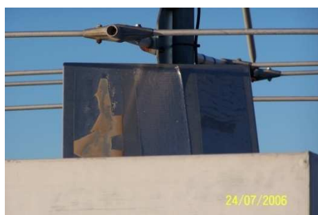
Figure 8.23. TP#1 taken 24 th July 2006, showing the almost total failure of the 3M substrate with wind causing the clear Mylar top layer to break-up, and showing failure of the Clear Dome substrate top right edge.
