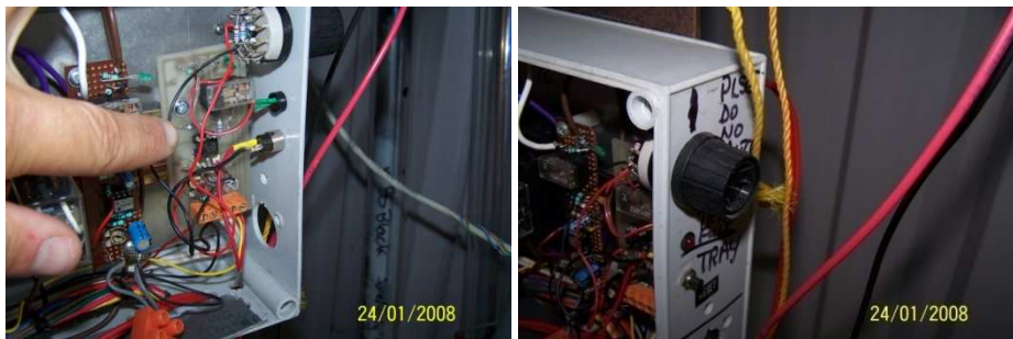
Figure 5.17 a & b. a) Tray full circuitry, b) Manual reset pushbutton and resistor adjustment.
