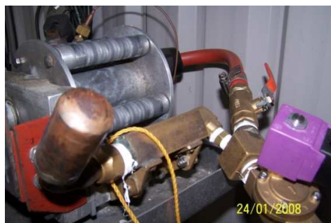
Figure 5.23. Inline filter and solenoid switch (from 2007).
