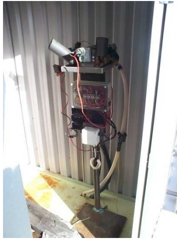
Figure 5.9. The original circulation pump.
