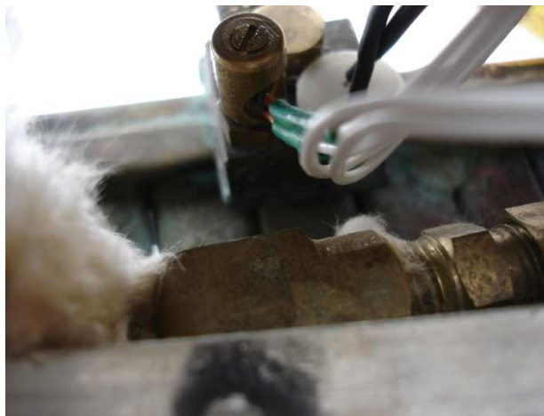
Figure 3.12. Showing the temperature and flow sensors as mounted.
