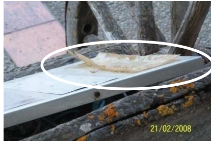
Figure 8.34. TP#2 taken in January 2008, as viewed from the rear of the panel.
