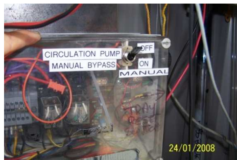
Figure 5.21. CP manual override bypass switch.
