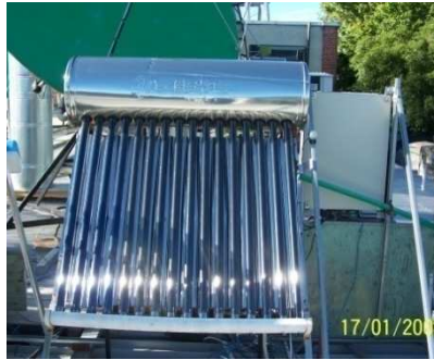
Figure 10.13. Solar batch collector.
