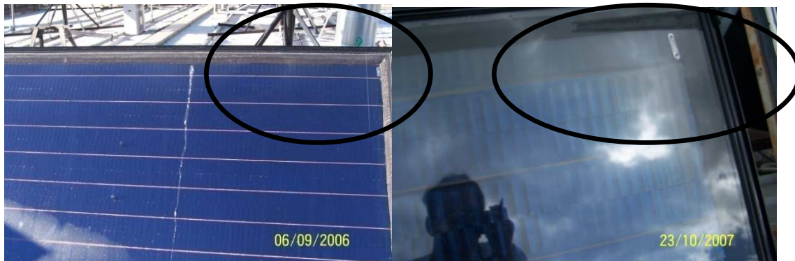
Figure 10.5 a & b. The urethane panel top right corner in Sept 2006 and Oct 2007, 13 months later.
