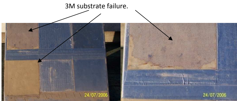
Figure 8.53 a & b. AP#1 taken 24 th July 2006, 3M substrate failure.
