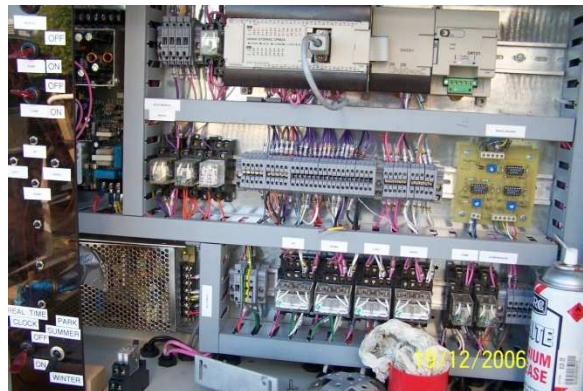
Figure 5.30. The control panel complete and in operation December 2006.
