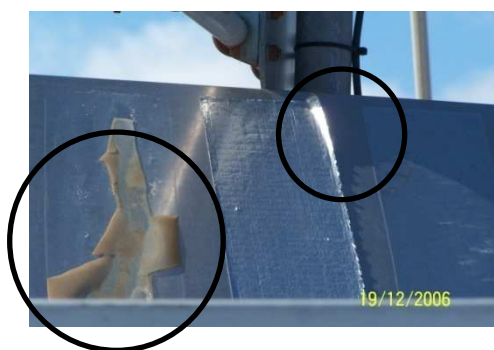
Figure 8.26. TP#1 taken 19 th December 2006, showing the lifting of the Clear Dome substrate, and total failure of the remaining 3M substrate.
