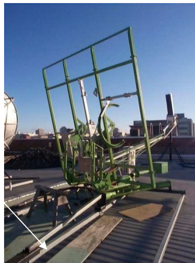
Figure 1.2. Rear 'Y' leg support with mounting adaptor bracket securing to satellite rail, mid 2003.
