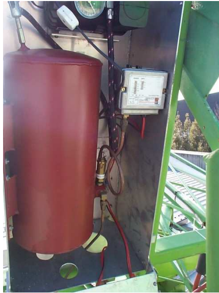
Figure 4.4. Air compressor and pressure vessel.
