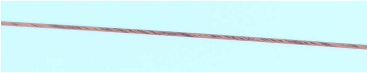
Figure 8 – Bungama transmission line conductor with a black substance apparently being emitted between strands.
