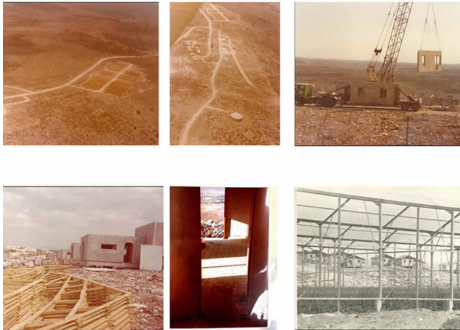
FIG. 3.10 Infrastructure works in Sal'it and Construction of Houses in Sal'it, 1980. (Smadar Gilboa) Note the “view” from the living room
