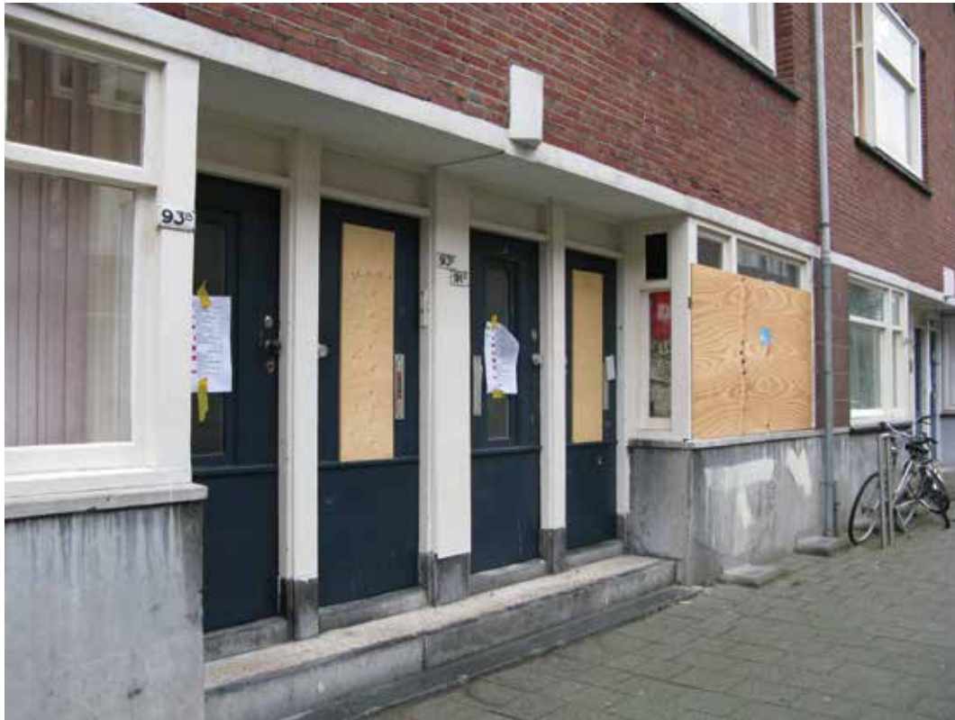
FIGURE 6.3 A property still vacant and in need of rehabilitation in 2009
