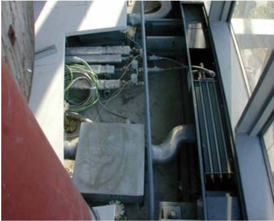
Figure 5.24 Decentralised ventilation components in a suspended floor; air and water supply lines are clearly visible
