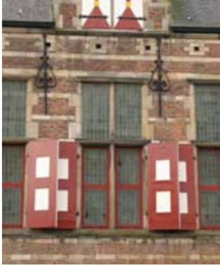
Figure 4.1: Dutch window; in early stages outfitted with folding shutters in the lower section to offer ventilation but provide rain tightness at the same time; and lead glazed window panes for lighting in the upper section.
