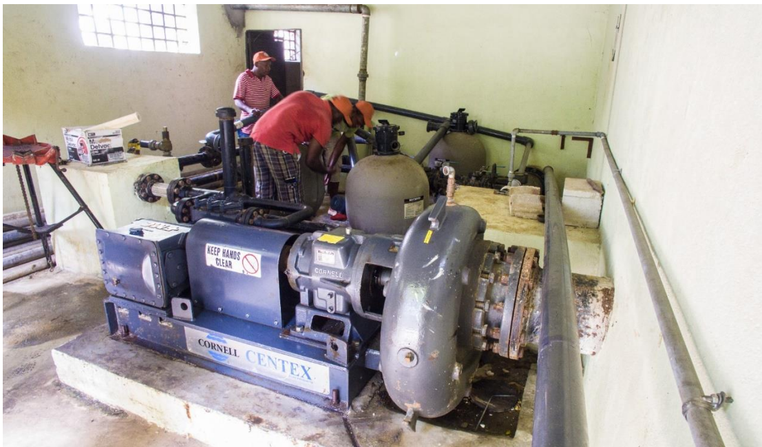
Figure 10. Example of the inside of one of the pump houses. Water flows through the turbine on the right and powers the piston pump on the left. Water from the turbine is discharged back into the stream outside the pumphouses that flows to Lake Peligre.
