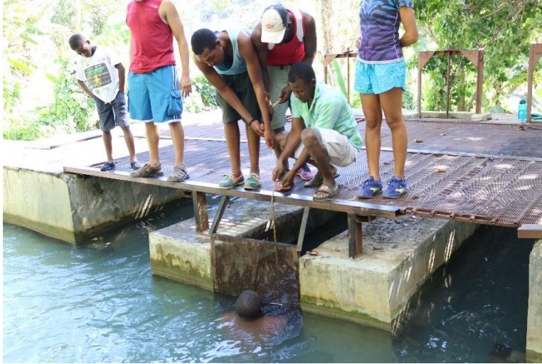
Figure 9. Image taken from behind the dam where the water flows into two penstocks that power the turbines.
