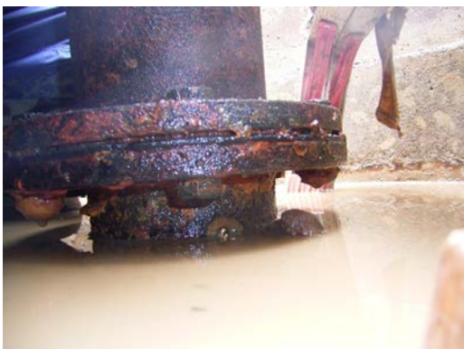
Photograph 2. Defect in air valve
