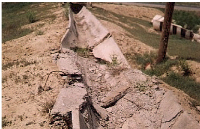
Figure 2. Deteriorated Irrigation Canal (Thurman, 2001)
