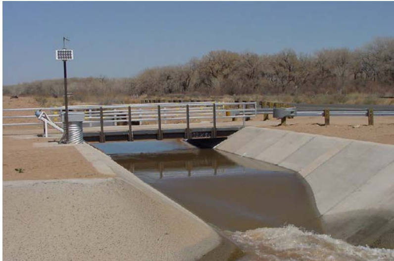
Figure 3. Broad Crested Weir Gauging Station with Radio Telemetry
