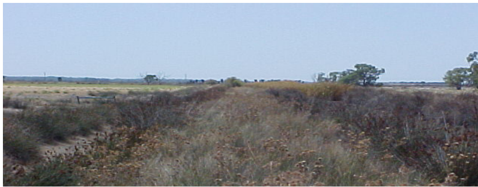
Photo 3. Low use supply channel infested with weeds
