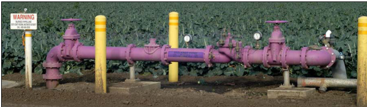
Figure 6. Irrigation Turnout on the South Pipeline
