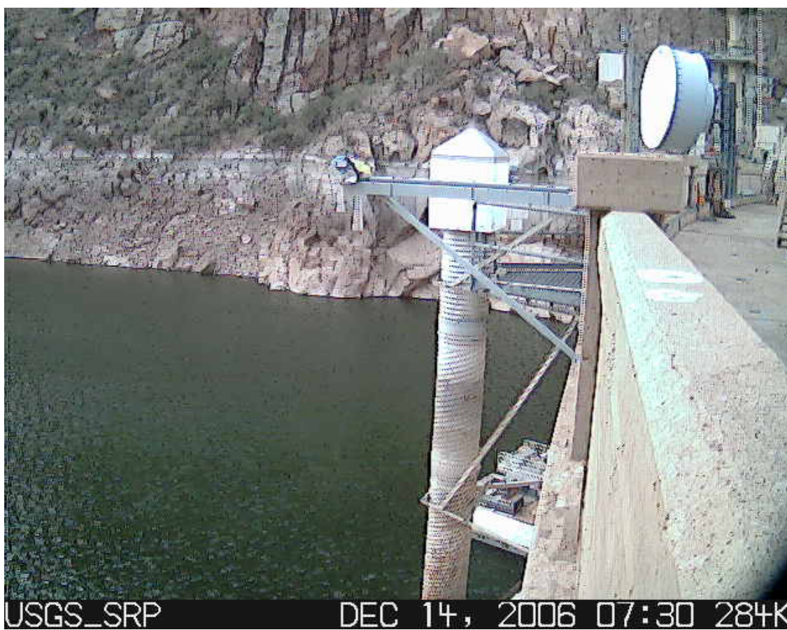
Figure 2. Photo of installed radars and stilling well at Horse Mesa Dam, Arizona, by digital camera attached to logger.
