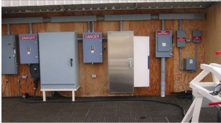
Figure 5. Electrical supply for the motor testing
