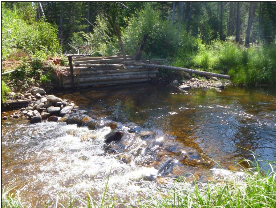
(B). Diversion of Beaver Creek at Rhea Ditch. Headgate composed of wooden logs with rock weir directing flow. Some water leaks through to ditch when headgate is closed.
