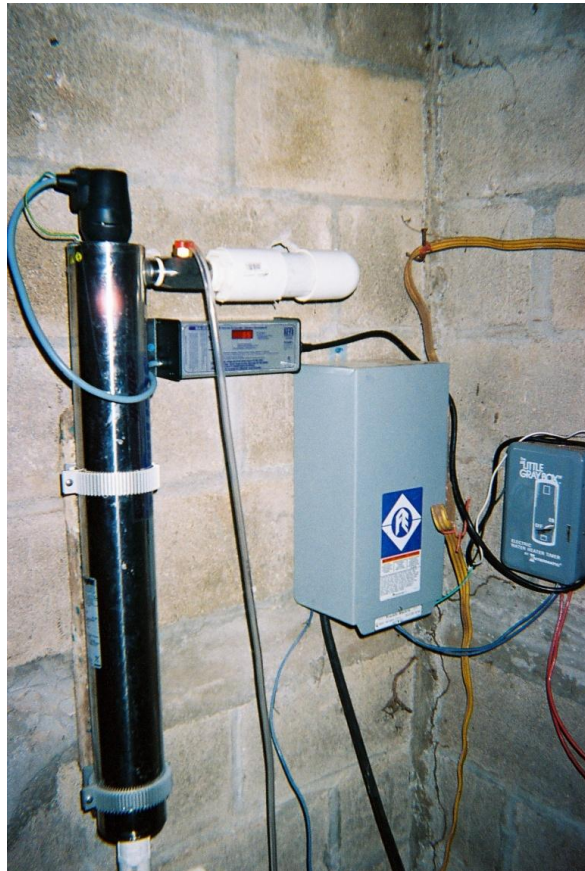
Figure 4.4 A UV disinfection system in Nueva Cajola, Guatemala
