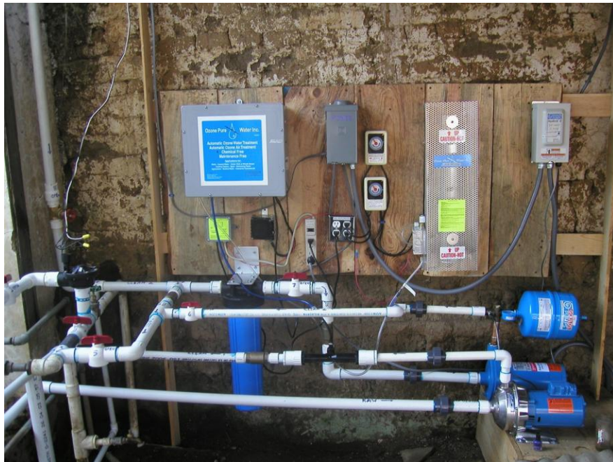
Figure 4.8 An ozone system near Quetzaltenango, Guatemala
