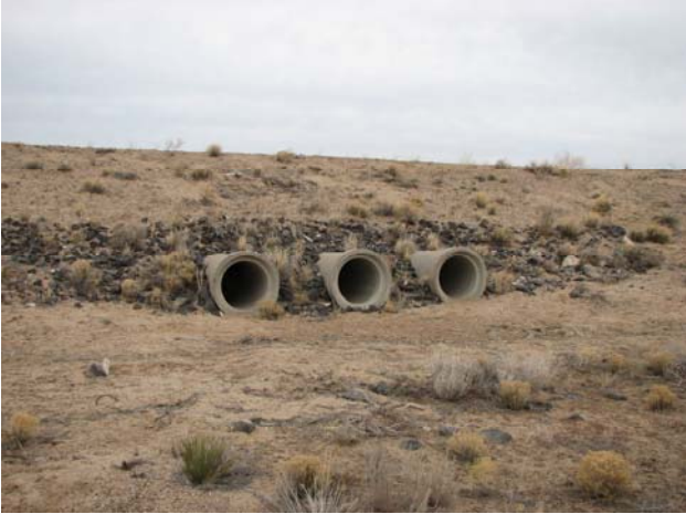
Ladera Dam System Managed by AMAFCA (Consisting of 15 dams.)
