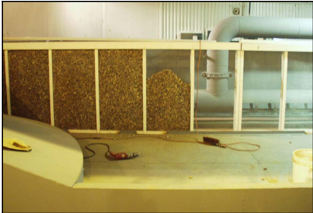
Figure 3.5: Headbox Under Construction Including Pipe Manifold and Rock Baffle (Figure 3.5 in Heintz (2002))
