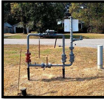
Figure 15 A Metering & Regulating (M&R) Facility.
