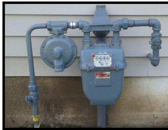
Figure 17 A Residential Customer Meter.
