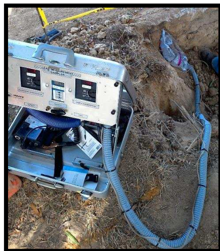
Figure 22 Exposed underground pipeline leak being measured using the INDACO high flow and plastic bag enclosure.
