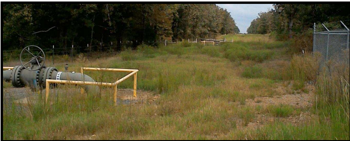
Figure 3 Gathering pipeline right of way(ROW) and block valve.
