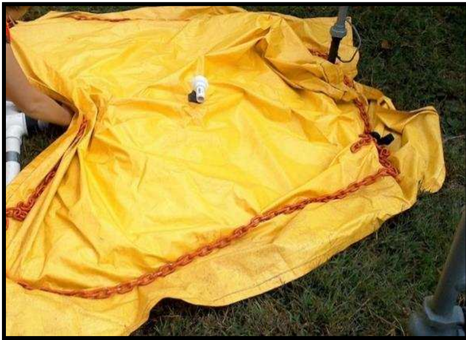
Figure 20 underground pipeline leak measurement enclosure. Placed over dead grass to capture leak diffusing through grass and along pipe that is connected to the above-ground pipe shown in the picture. Chain is used to provide a loose seal over the enclosure.
