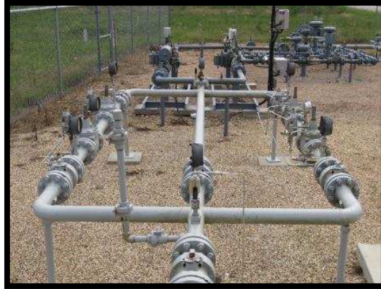
Figure 16 A Transmission Distribution Transfer Station (TDTS).
