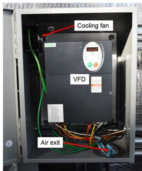
Figure 4-37. Tunnel circulation fan variable frequency drive.
