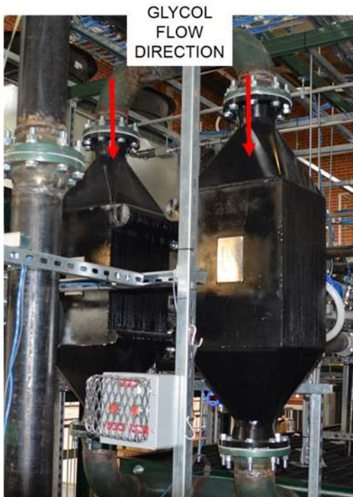
Figure 4-21. Chillers installed in facility.
