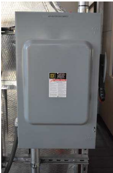
Figure 4-69. Air heater disconnect switch.
