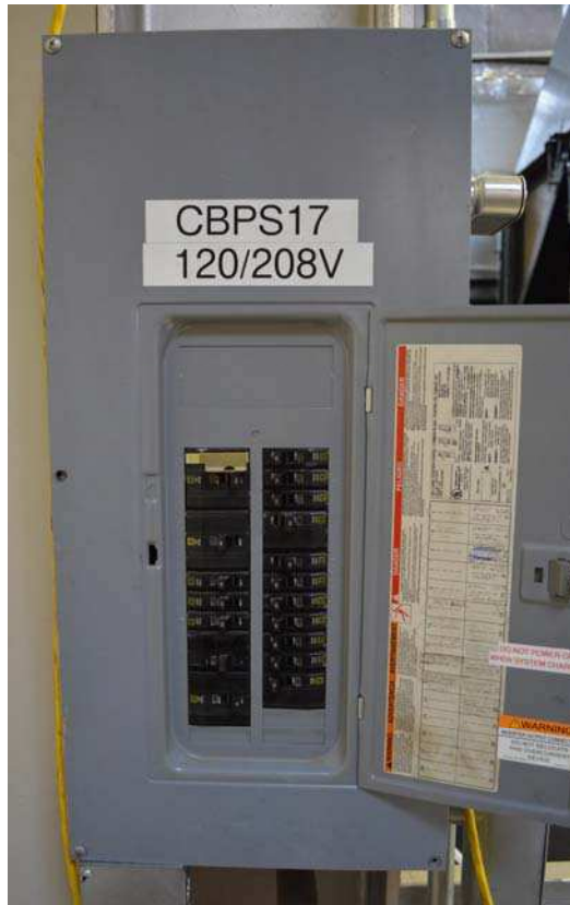
Figure 4-70. 120VAC powerhouse distribution panel.
