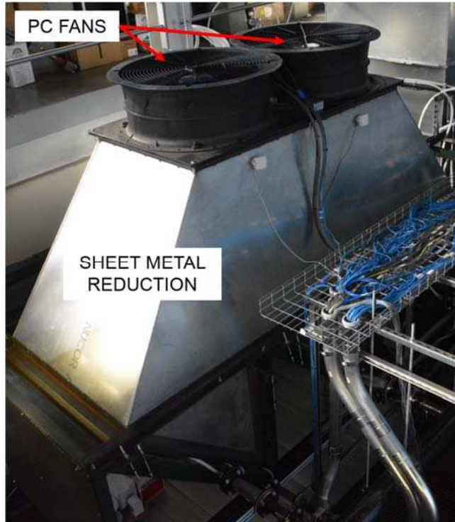
Figure 4-18. PC condenser cooling tower.
