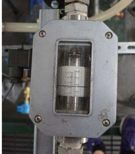
Figure 4-79. Bearing drain line volumetric flow meter.
