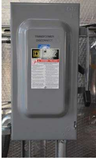
Figure 4-67. Transformer disconnect switch.
