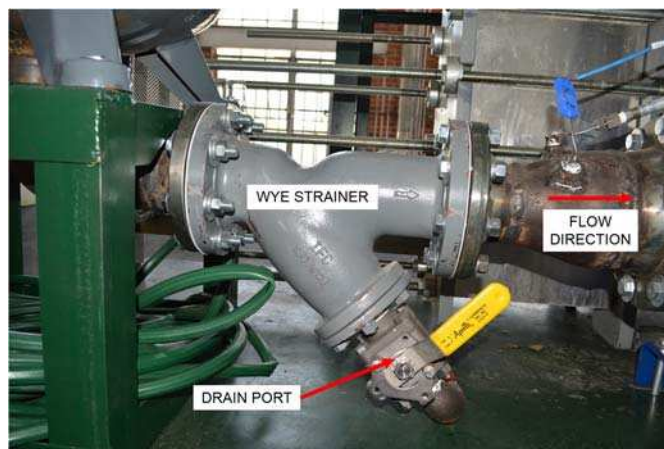
Figure 4-41. Glycol loop wye strainer.
