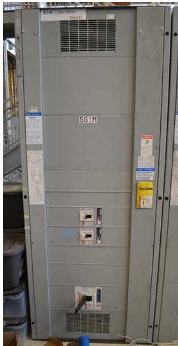
Figure 4-65. Switchboard for the TCCS.
