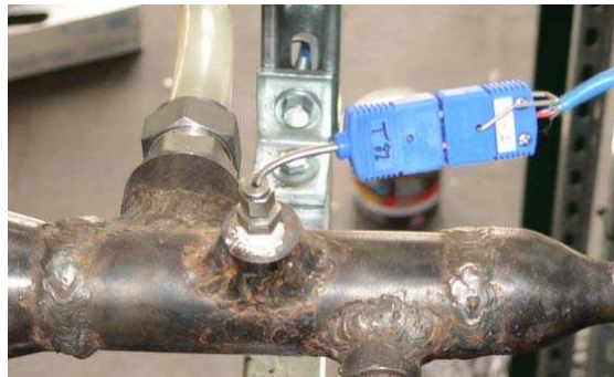
Figure 4-73. Thermocouple in pipe.
