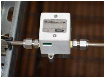
Figure 4-80. Bearing inlet volumetric flow meter.
