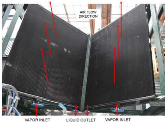
Figure 4-27. Cooling cycle condensers in one rack prior to complete installation.
