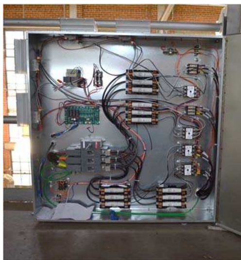
Figure 4-35. Heater control panel with inputs from Labview program.
