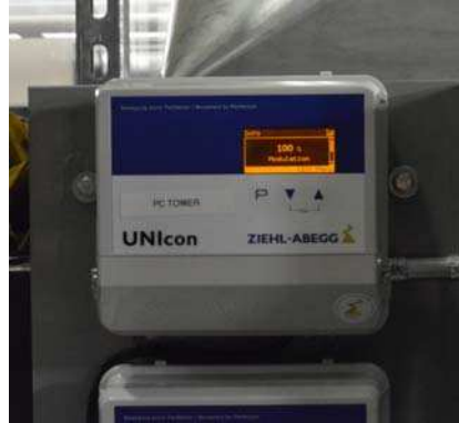
Figure 4-19. UNIcon Modbus master control unit for condenser fans.
