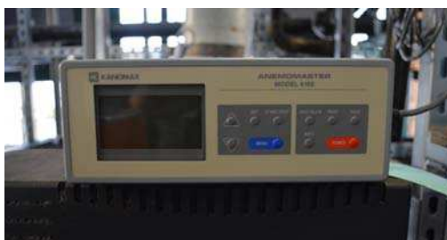
Figure 4-77. Kanomax anemomaster control module and LCD display.
