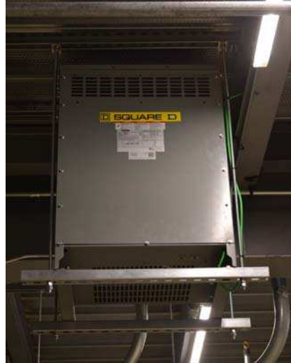
Figure 4-68. Transformer located beneath the mezzanine.
