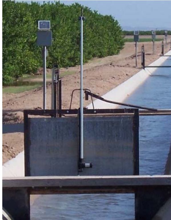
Figure 3. Actuator on Ditch Check Gate with Field Turnouts in Background
