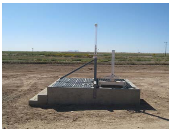
Figure 4. Pipeline Lateral Turnout
