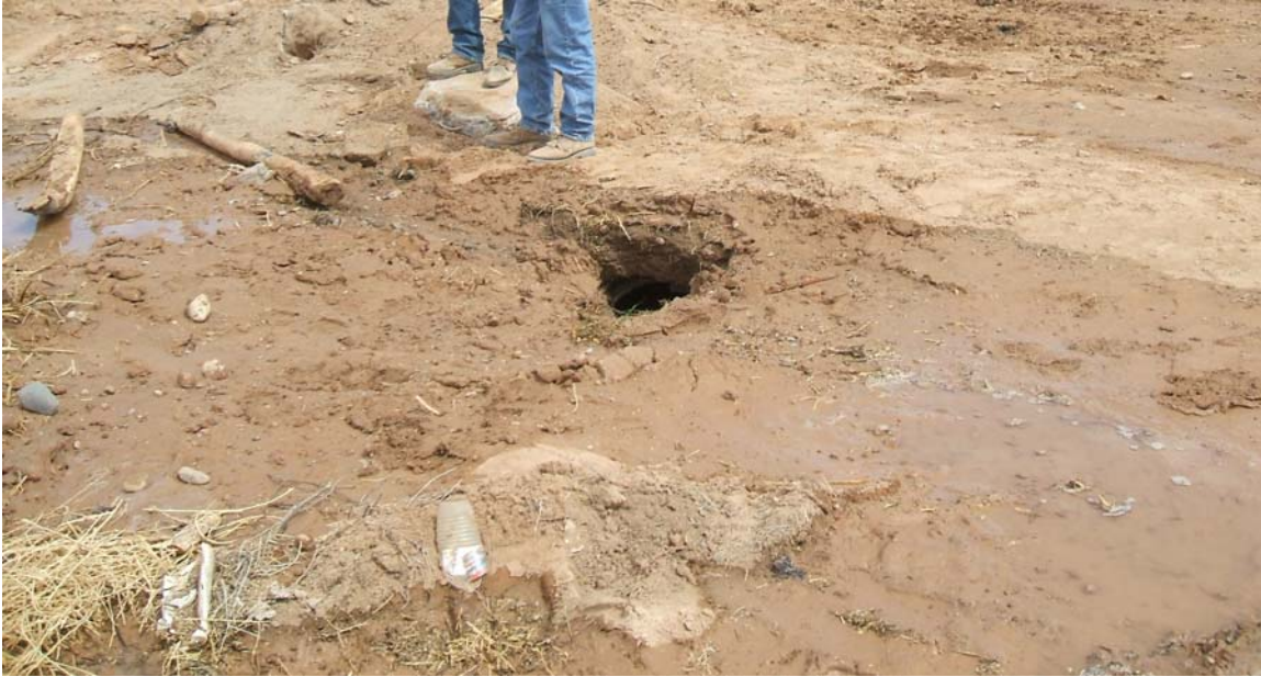
Figure 2. Broken Pipe Section
