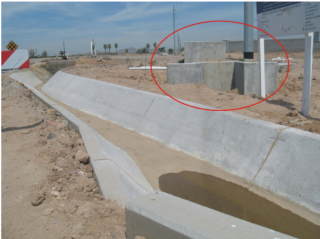
Figure 5. Abandoned structures waiting for a connection to the lateral
