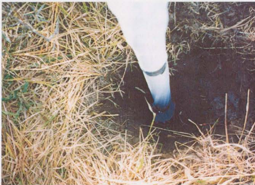
Figure 3.10. Installation of Well E. Done on September 20, 2003. The hole was backfilled after this picture was taken (the well, thought here to be installed on a bank, was later submerged by a spring).
