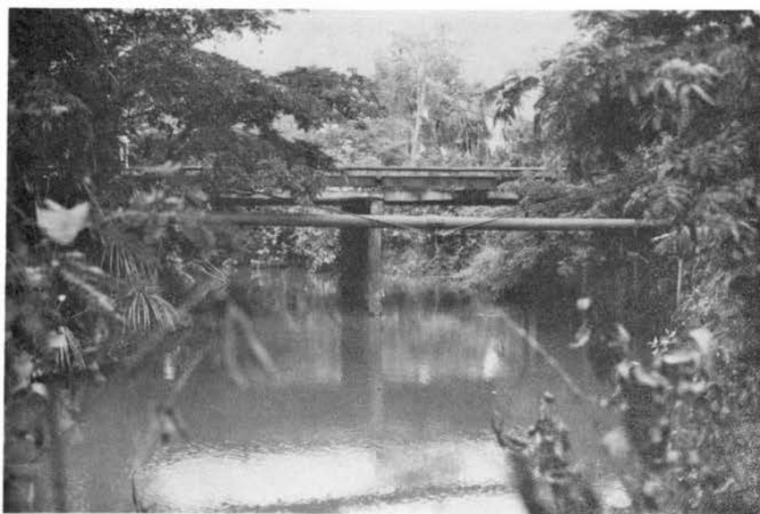
View looking downstream to the bridge over the Río Aisme. The SR recorder is visible on the left side of the photograph.
