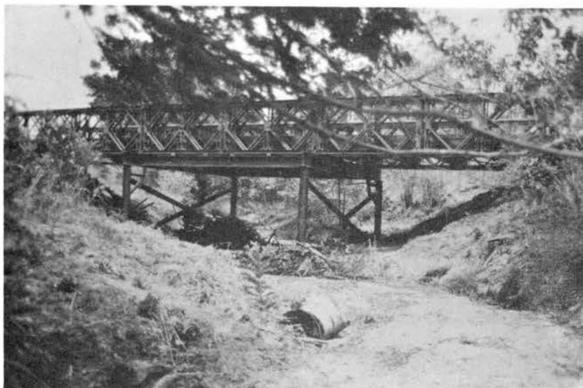
View looking downstream to the bridge over the Río Chupururo near Campo Mata. The float well for the SR recorder is visible between the cross-bracing on the right set of piers.
