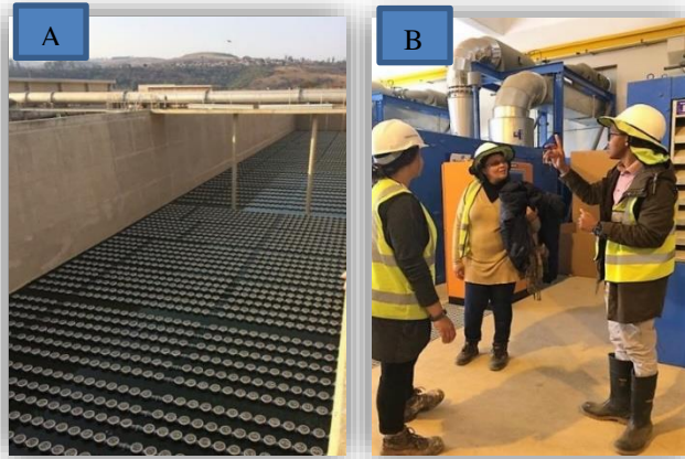
Figure 3.11: Recently installed (A) coarse-bubble air diffuser in aeration tank and (B) aeration blower at Darvill Treatment Works in Pietermaritzburg, South Africa. Pictures from site tour in 2017.
