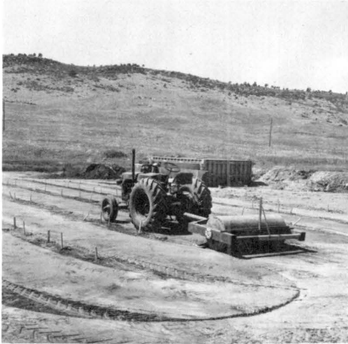
Fig. 7. A special steel roller was constructed for compaction between the 100" cross sections
