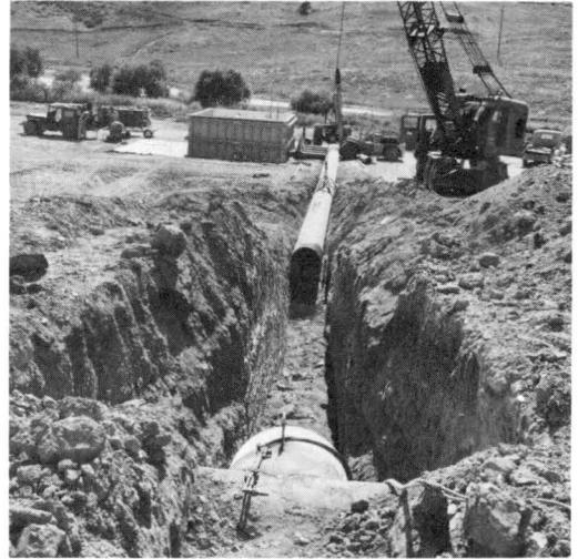
Fig. 12. Installation of the 24-inch line between the main supply line and headbox required a considerable amount of excavation in very resistant material
