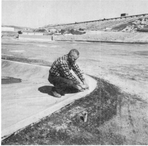
Fig. 19. The top of the dam was finished to the proper elevation with a "masons stone"
