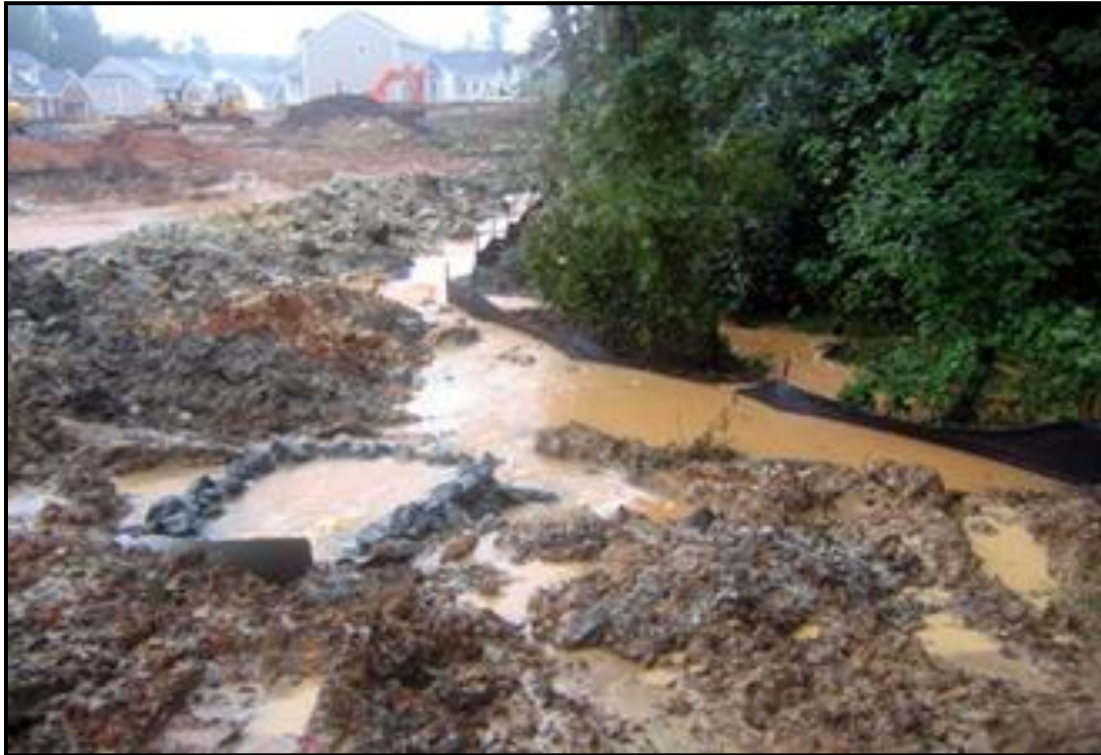
Figure 1.1 – Example of construction site erosion and sediment issues
