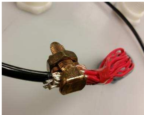
Figure 9 Exterior of reactor, 12-gauge wires joined with 2-gauge wires using split bolt connector, shown unwrapped. Cord grip is in untightened state
