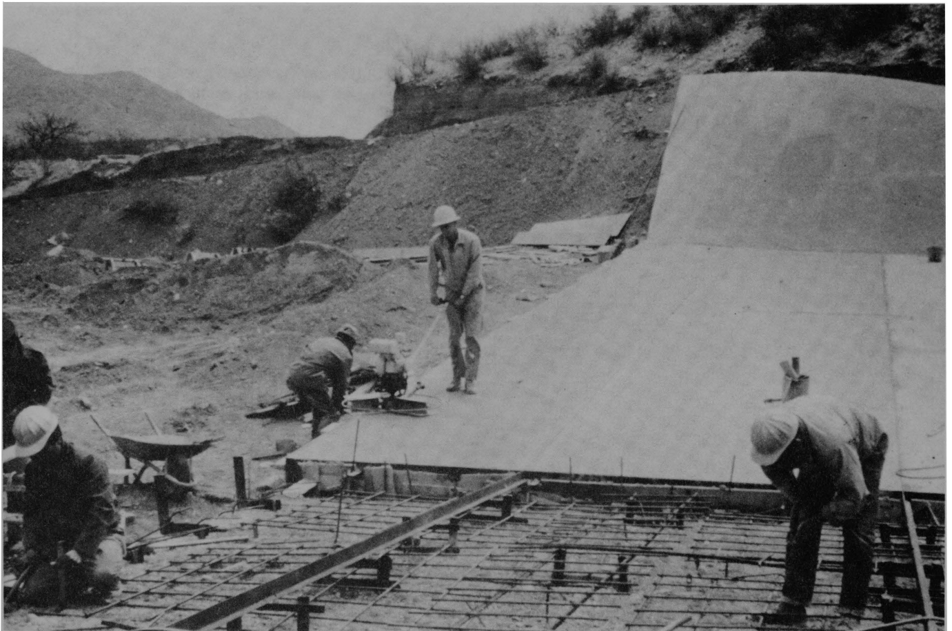
FIGURE 43.—Flume construction showing pouring of the floor area with screed controls in the foreground.
