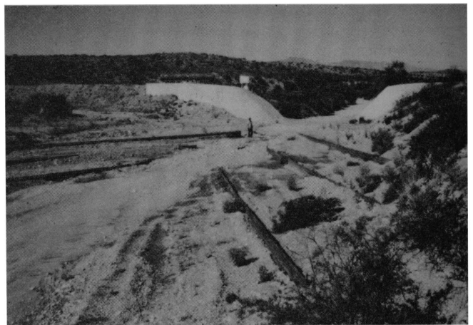
FIGURE 32.—Control dikes in place above flume 63.011, Walnut Gulch Watershed. BN-48661
