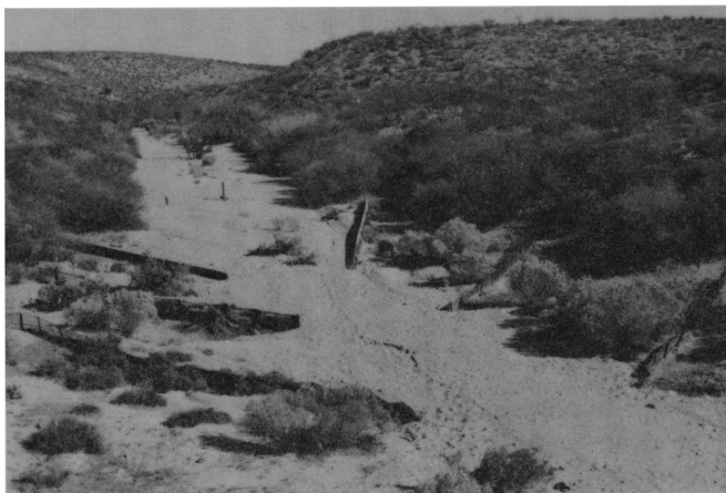
FIGURE 31.—Prototype control dikes at flume 63.003 after large storm flow in early dike evaluation at Walnut Gulch Watershed. BN-48660
