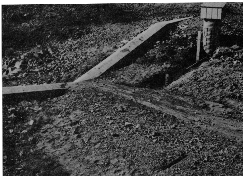
FIGURE 1.— V -notch concrete weir filled with bed-load near Stafford, Ariz.
