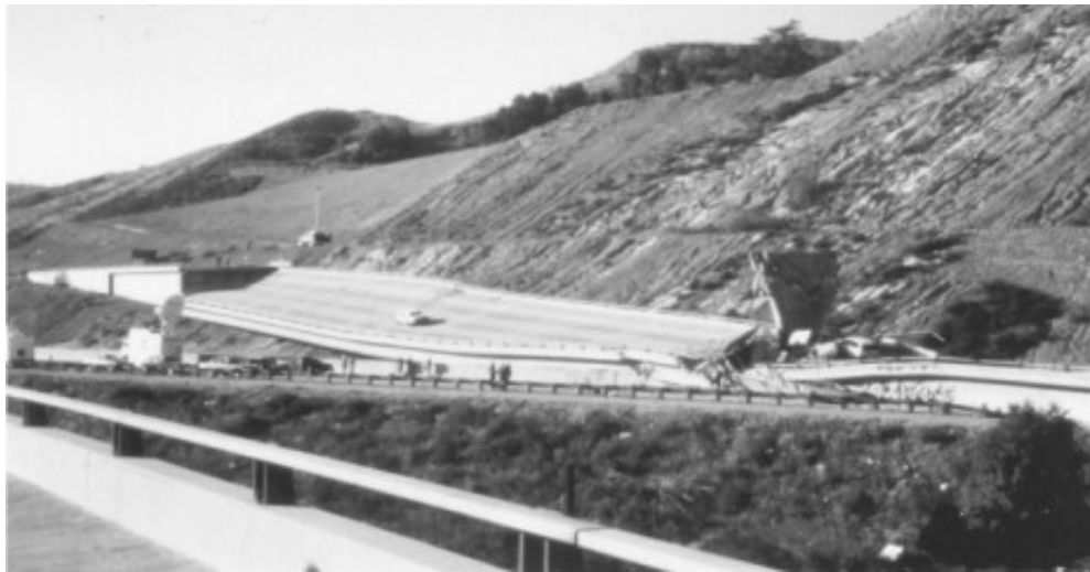
Figure 2.6 (Earthquake Engineering Research Institute (EERI), 1996) South Connector Overcrossing Failure
