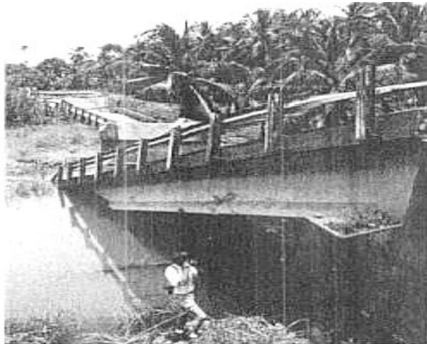
Figure 2.5 (Cole, 1991). Costa Rica Earthquake, Rio Bananito Bridge Failure.
