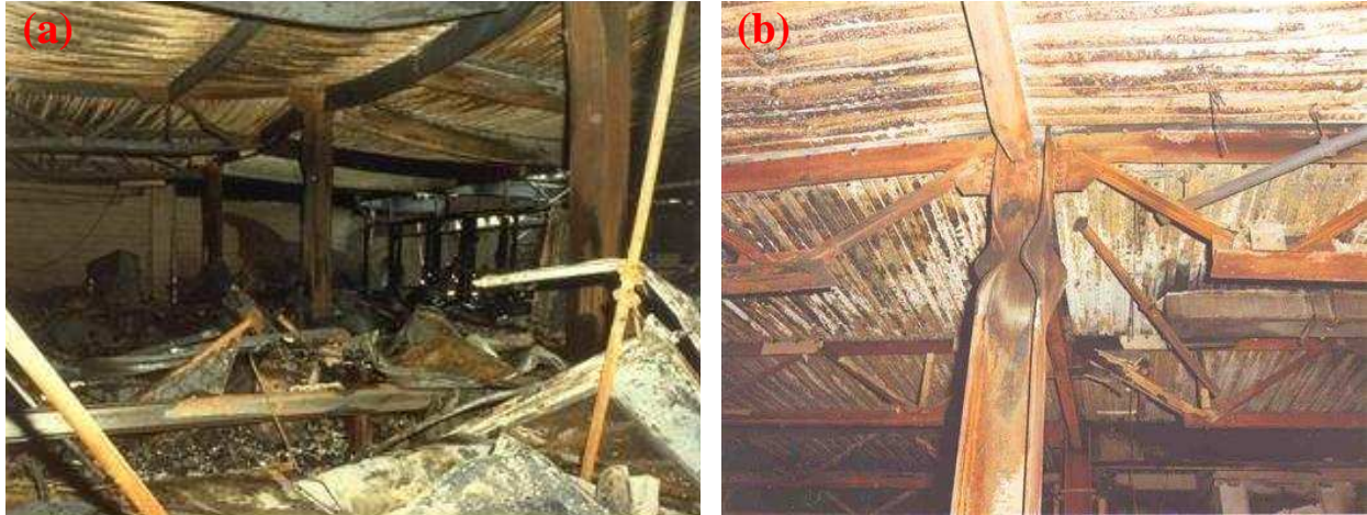
Figure 2.7 (a) Large permanent deflections in composite beams and trusses and (b) significant local buckling in flanges and web of a steel column in Broadgate project (Broadgate phase 8) fire.
