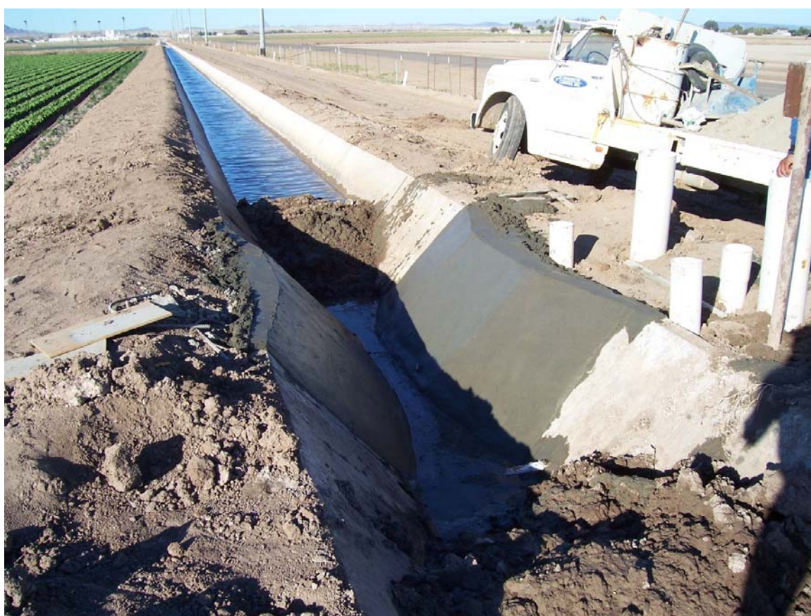
Figure 3. University of Arizona Valley Farm submerged flume site
