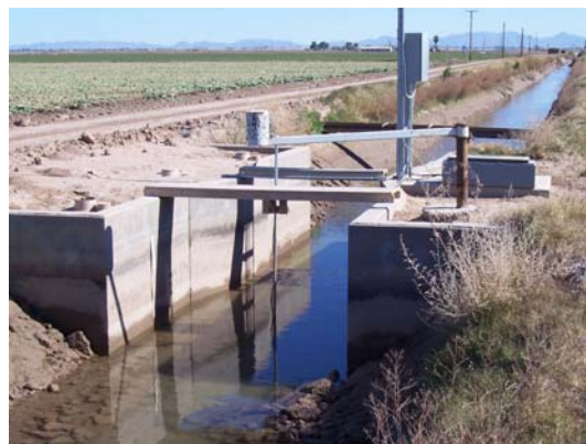
Figure 9 ADFM unit at Cumming Flume
