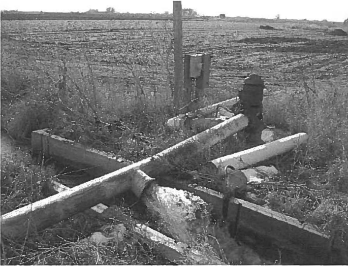
Figure 3. Retiming well in operation. Water is pumped from the ground and is delivered to the river to cover stream depletions from irrigation well pumping. Sometime in the near future, stream depletions from the retiming well will occur in the river, and must be covered.
