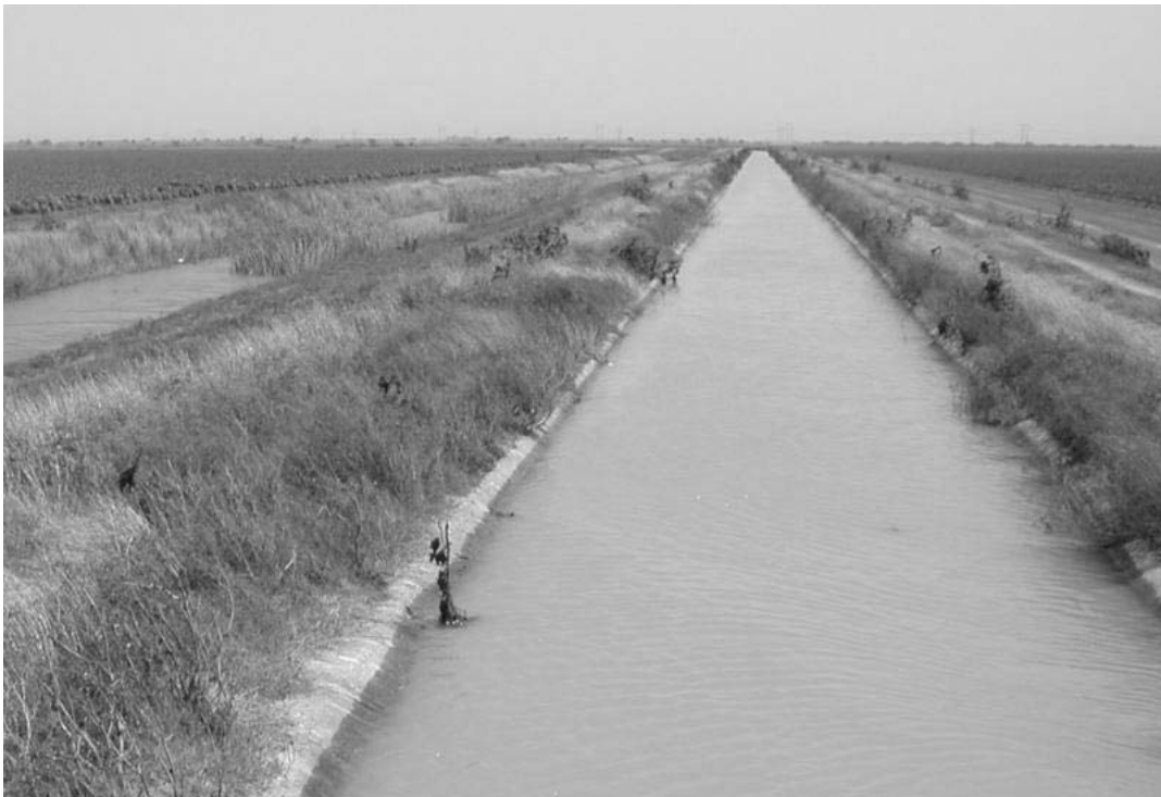
Photo 2. Example of Seepage Adjacent to Cracked Concrete Irrigation Canal
