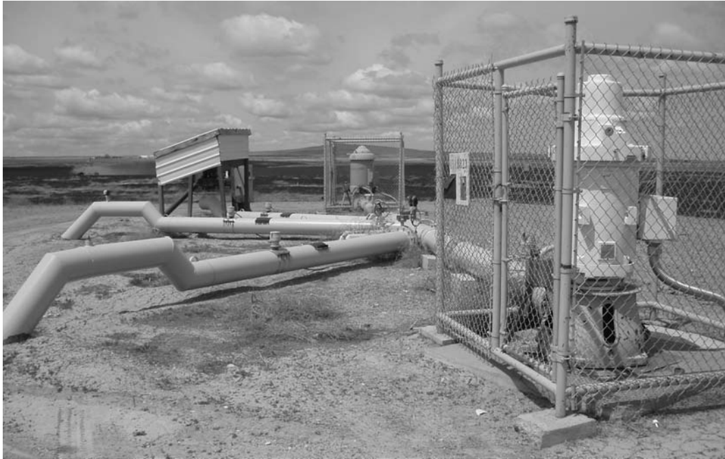
Figure 3. Two district supply wells directly coupled to three metered farm deliveries. The well at the right has VFD to regulate pressure. A farm booster pump is installed under shade at left.
